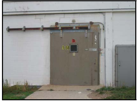
Secured Access Door Outside of Biocontainment
