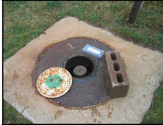
Manhole Cover to Underground
