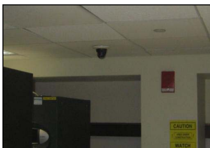
Server Room Security Camera
