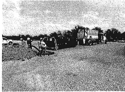
Photo #8 View of the vacuum truck and associated storage container.
