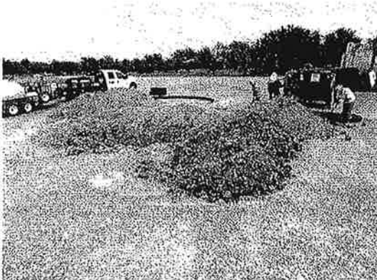
Photo #9 View of the excavated soil being loaded into the vacuum truck and associated storage container.
