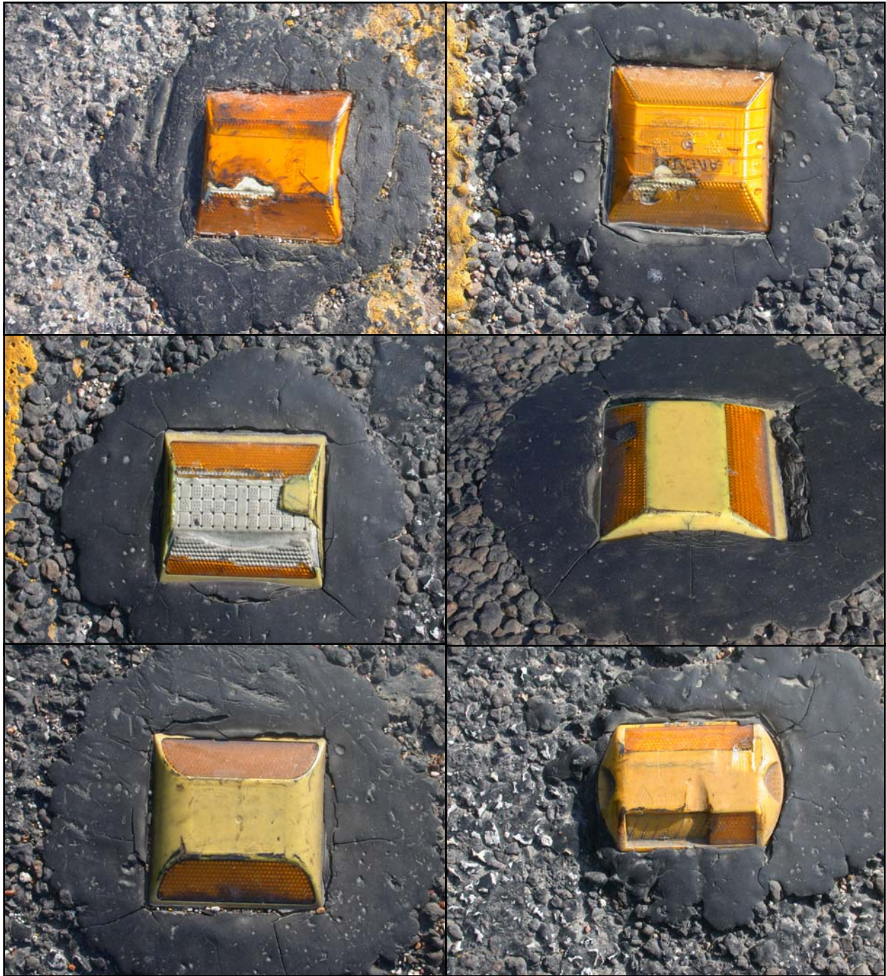
Figure 90. Typical RRPM Damage on Seal Coat Pavement in Bryan.
