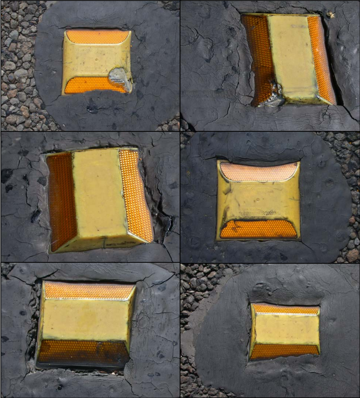
Figure 87. Typical RRPM Damage on Seal Coat Pavement in Lufkin.
