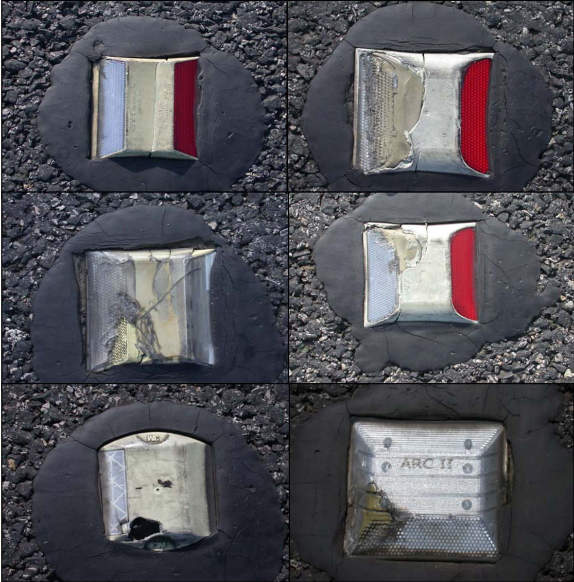
Figure 78. Typical RRPM Damage on Asphalt Pavement in Rural Laredo.
