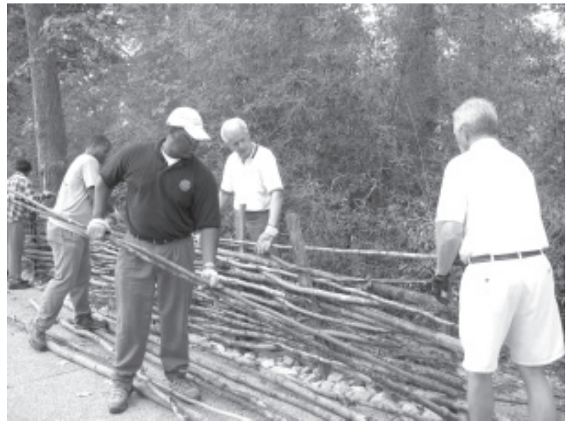
Members of the James City County Rotary Club constructed wattle fencing at Jamestown Settlement.
