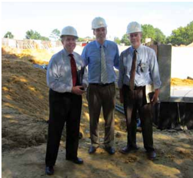
U.S. Senator Mark Warner (center) came to the Yorktown Victory Center September 5 for a tour and briefing on the American Revolution Museum at Yorktown. He is shown at the construction site of the new museum building with Jamestown-Yorktown Foundation Executive Director Phil Emerson and Acting Senior Director of Museum Operations and Education Jim Holloway.
