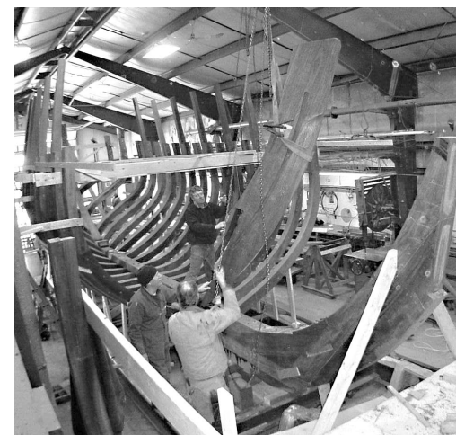
Shipwrights at Boothbay Harbor Shipyard hoist the last stem piece into position on the frame of the Discovery .
