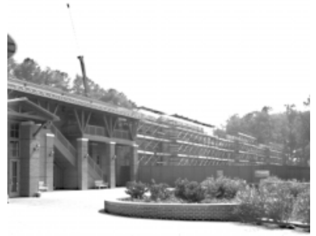
The permanent gallery exhibit building under construction adjoins the new theater and special exhibition wing.
