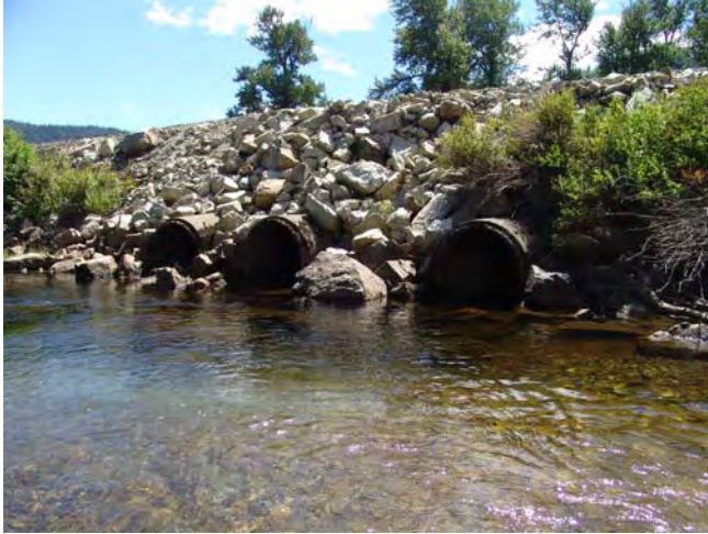
Figure 7. View to the south near RM 9.7 looking at the right river bank with concrete culvert invert at water surface level. (Reclamation photograph by D. Bennett, August 8, 2007).
