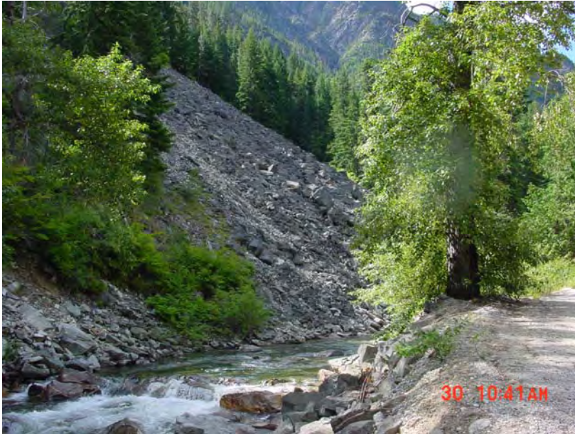
Figure 6. Example of slope failure on right side of river just upstream of White Pine Railroad Bridge. (Reclamation photograph taken by J. Bountry, June 2005).
