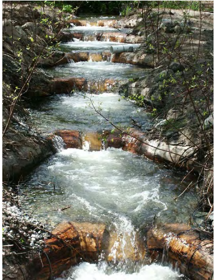
Photo A-18. Looking upstream at the six weirs that have replaced the Mill Creek Diversion and restored fish passage.
