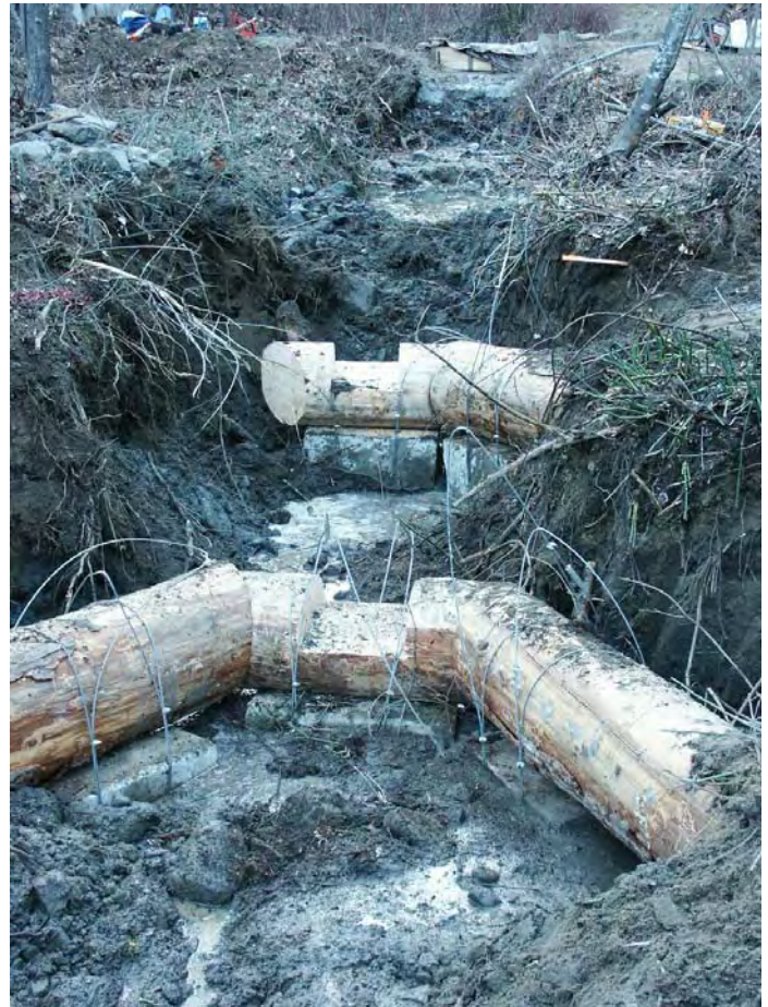
Photo A-10. Weir No. 6 fully installed; Weir No. 5 with center piece and left arm is in place.
