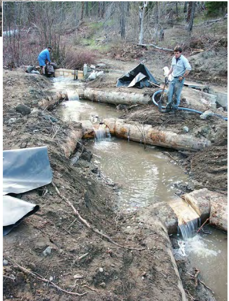
Photo A-14. The bypass has been closed and "first water" flows through the new weirs on Mill Creek; note lack of clarity of water clouded by sediment.
