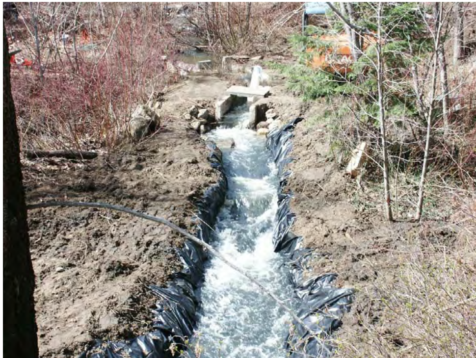
Photo A-4. Diverting water through temporary bypass channel; note use of polyethylene liner to limit erosion.
