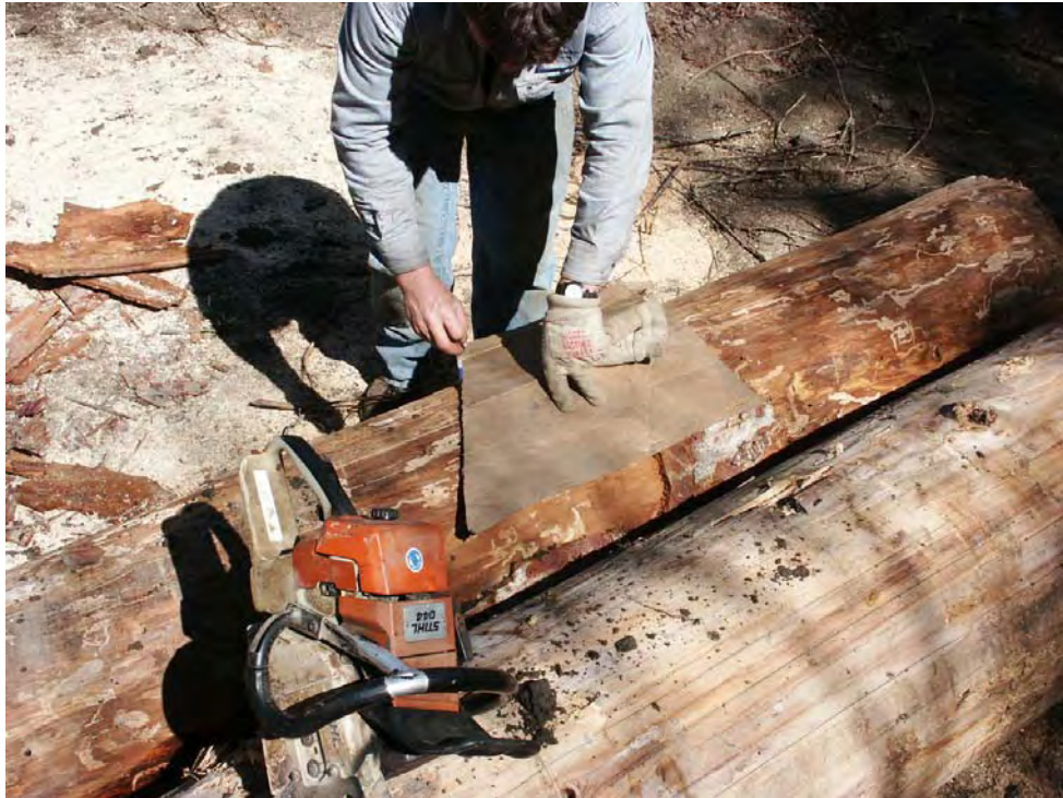
Photo A-5. Preparing to cut logs for weir arm. The template was used to ensure the proper angle for butting the ends of the logs.
