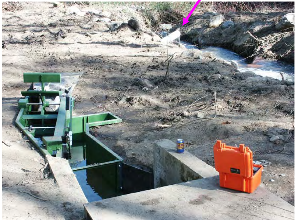
Photo A-16. The new fish screen was purchased under a FRIMA grant through WDFW. The arrow indicates the outflow of the bypass pipe .
