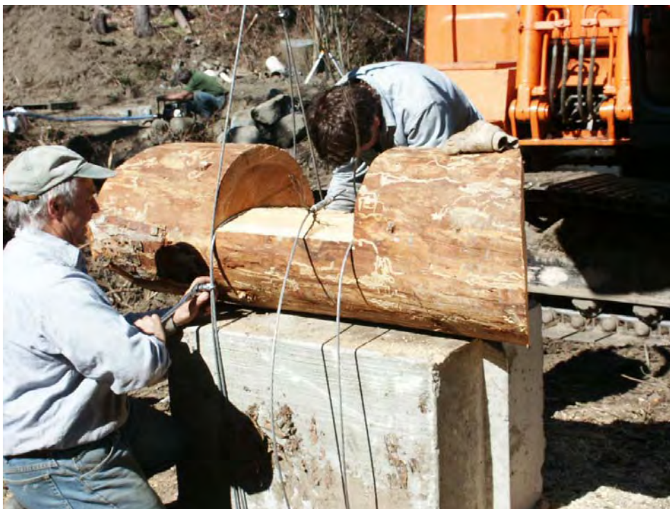
Photo A-6. Workers use cable to secure the weir's notched, low-flow center crosspiece.
