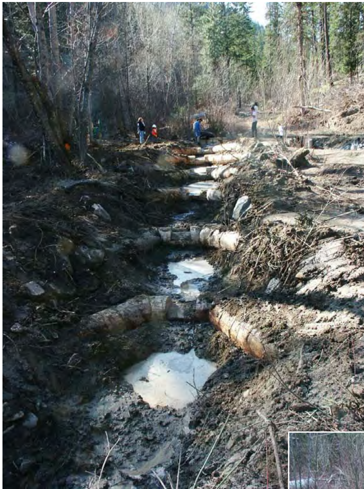
Photo A-13. Looking upstream at completed weirs; groundwater has filled the individual scour holes.
