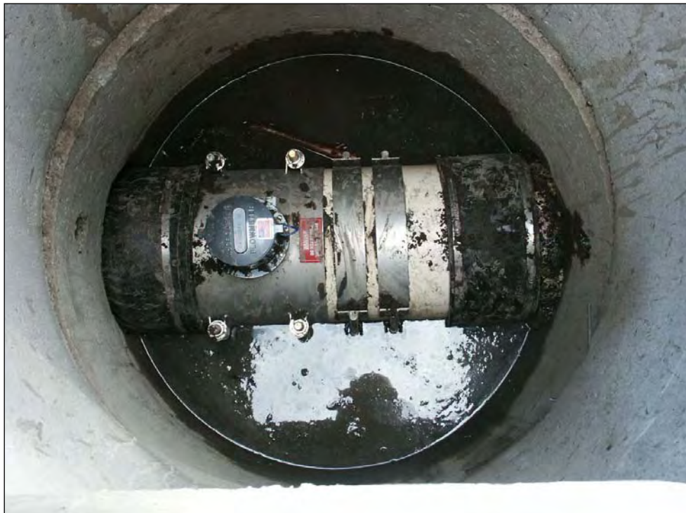
Photo A-21. Flow meter installed downstream from the diversion structure near the point-of-diversion.
