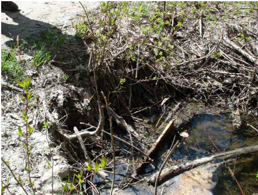
Photograph No. 3. View of the intake of a culvert that drains a wetland area. Kahler Reach; Subreach OZ-3, Nason Creek - Wenatchee Subbasin, Washington. Bureau of Reclamation Photograph by R. McAfee, May 4, 2007.
