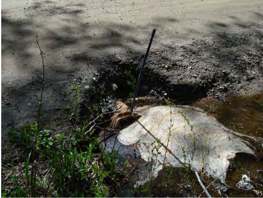
Photograph No. 2. View showing the top end of a culvert that drains a wetland area. Kahler Reach; Subreach OZ-3, Nason Creek - Wenatchee Subbasin, Washington. Bureau of Reclamation Photograph by R. McAfee, May 4, 2007.
