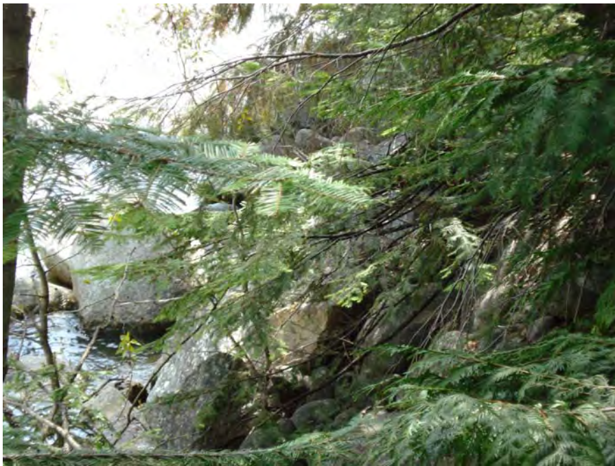
Photograph No. 10. View to the east of riprap along the toe of the road base on the right bank. Kahler Reach; Subreach IZ-4, Nason Creek - Wenatchee Subbasin, Washington. Bureau of Reclamation Photograph by R. McAfee, May 7, 2007.
