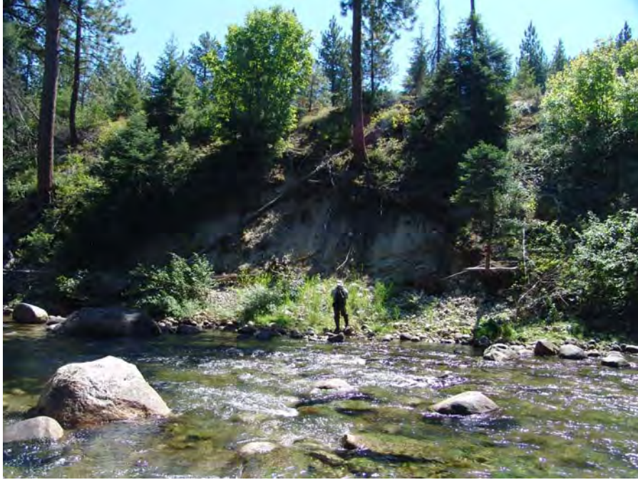
Photograph No. 2. View is to the east showing erosion along a tall terrace that forms the right bank. Kahler Reach; Subreach IZ-2, Nason Creek - Wenatchee Subbasin, Washington. Bureau of Reclamation Photograph by D. Bennett 8/9/07.
