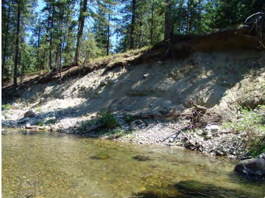
Photograph No. 6. View is to the northeast looking downstream showing erosion of the tall terrace along the right bank. Composition is a mixture of sand and gravel with cobbles. Kahler Reach; Subreach IZ-2, Nason Creek - Wenatchee Subbasin, Washington. Bureau of Reclamation Photograph by D. Bennett 8/9/07.
