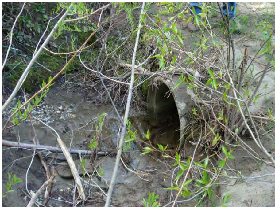
Photograph No. 1. View of the east (wetland) side of a culvert. Kahler Reach; Subreach DIZ-2, Nason Creek - Wenatchee Subbasin, Washington. Bureau of Reclamation Photograph by R. McAfee, May 5, 2007.
