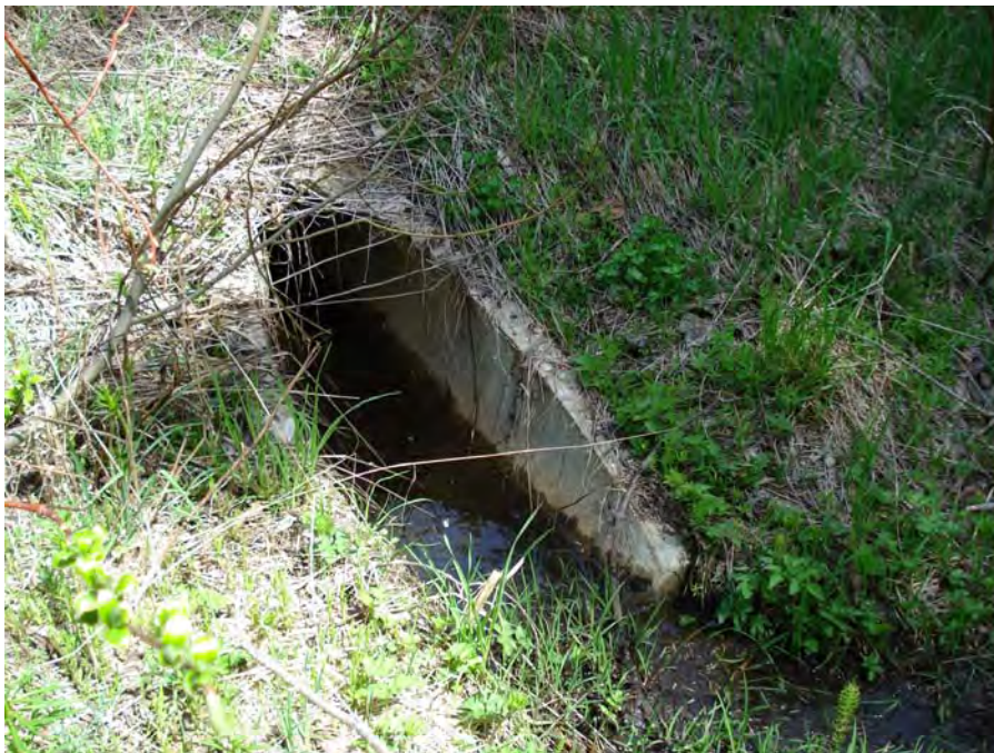
Photograph No. 1. Concrete culvert at the upstream end of a historic oxbow located to the south of U.S. Highway 2.. Kahler Reach; Subreach DIZ-1, Nason Creek - Wenatchee Subbasin, Washington. Bureau of Reclamation Photograph by R. McAfee, May 7, 2007.
