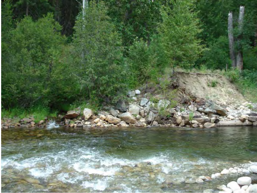
Photograph No. 151. View from the right bank looking to the north showing a channel unit sequence of rapid to scour pool with an old bridge abutment and stream/wetland inlet along the left bank of the river. Kahler Reach; Subreach IZ-4, Nason Creek - Wenatchee Subbasin, Washington. Bureau of Reclamation Photograph by R. M o Affee, August 12, 2007.
