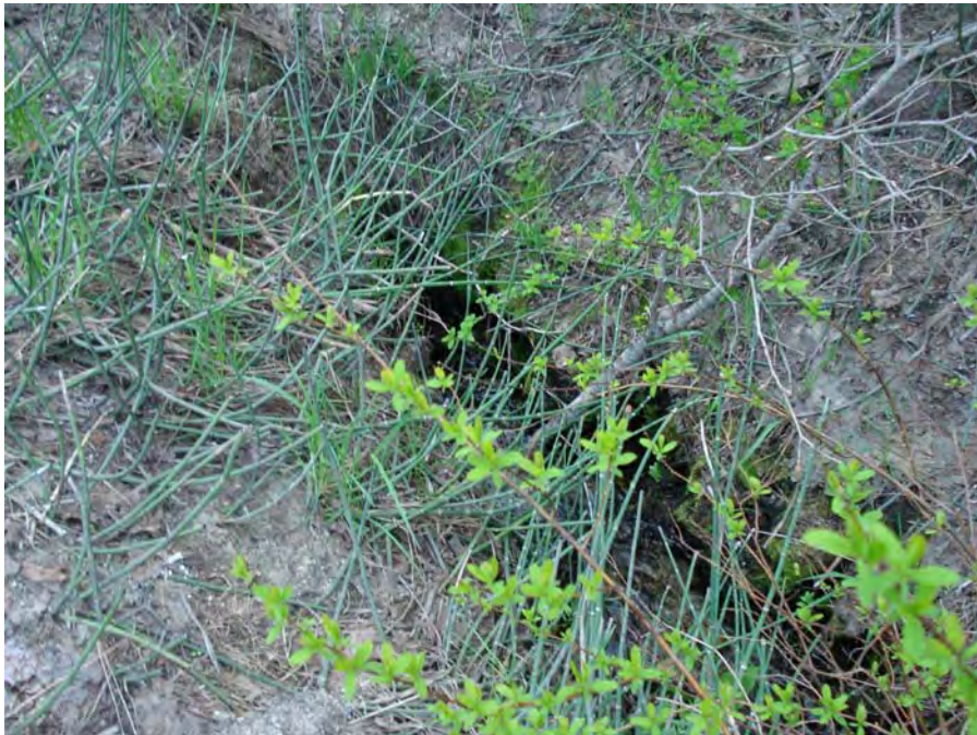
Photograph No. 3. Intake of culvert that drains wetlands in the lower section of historic oxbow located to the south of U.S. Highway 2. Kahler Reach; Subreach DIZ-1, Nason Creek - Wenatchee Subbasin, Washington. Bureau of Reclamation Photograph by R. McAfee, May 7, 2007.
