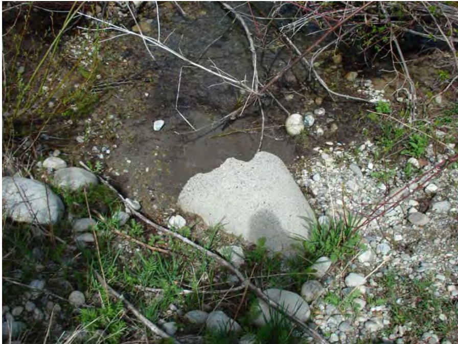
Photograph No. 20. View of the west (river) side of a culvert. Kahler Reach; Subreach IZ-4, Nason Creek - Wenatchee Subbasin, Washington. Bureau of Reclamation Photograph by R. McAfee, May 5, 2007.
