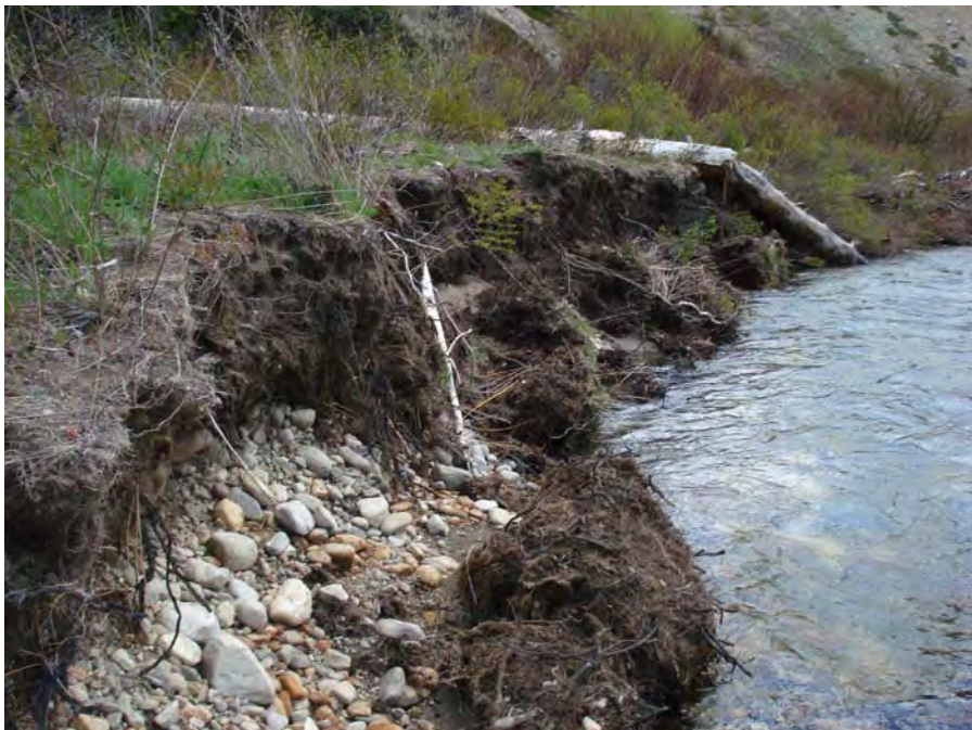
Photograph No. 13. View to the southeast showing local erosion along the left bank. Composition is a mixture of sand with gravel and cobble. Kahler Reach; Subreach IZ-2, Nason Creek - Wenatchee Subbasin, Washington. Bureau of Reclamation Photograph by R. McAfee, May 4, 2007.
