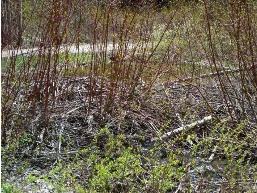
Photograph No. 4. View showing the outfall of the culvert and wetlands, with another culvert in the road embankment in the back ground. Kahler Reach; Subreach OZ-3, Nason Creek - Wenatchee Subbasin, Washington. Bureau of Reclamation Photograph by R. McAfee, May 4, 2007.
