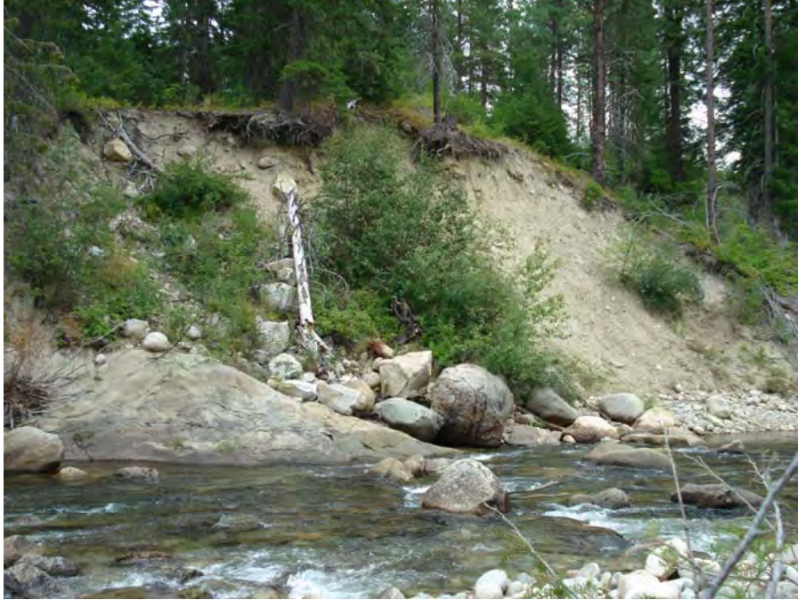
Photograph No. 5. View from the right bank looking to the southeast showing a bedrock outcrop, boulders and landslide along the left bank of the river. Kahler Reach; Subreach IZ-4, Nason Creek - Wenatchee Subbasin, Washington. Bureau of Reclamation Photograph by R. M o Affee, August 12, 2007.
