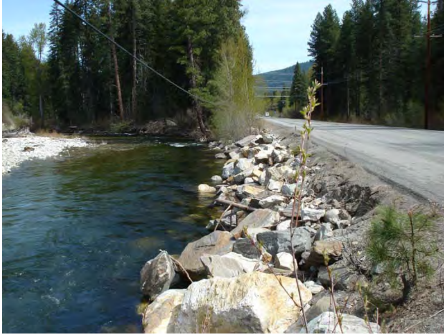
Photograph No. 17. View to the north of a scour pool associated with riprap along the base of the highway. Kahler Reach; Subreach IZ-4, Nason Creek - Wenatchee Subbasin, Washington. Bureau of Reclamation Photograph by R. McAfee, May 5, 2007.
