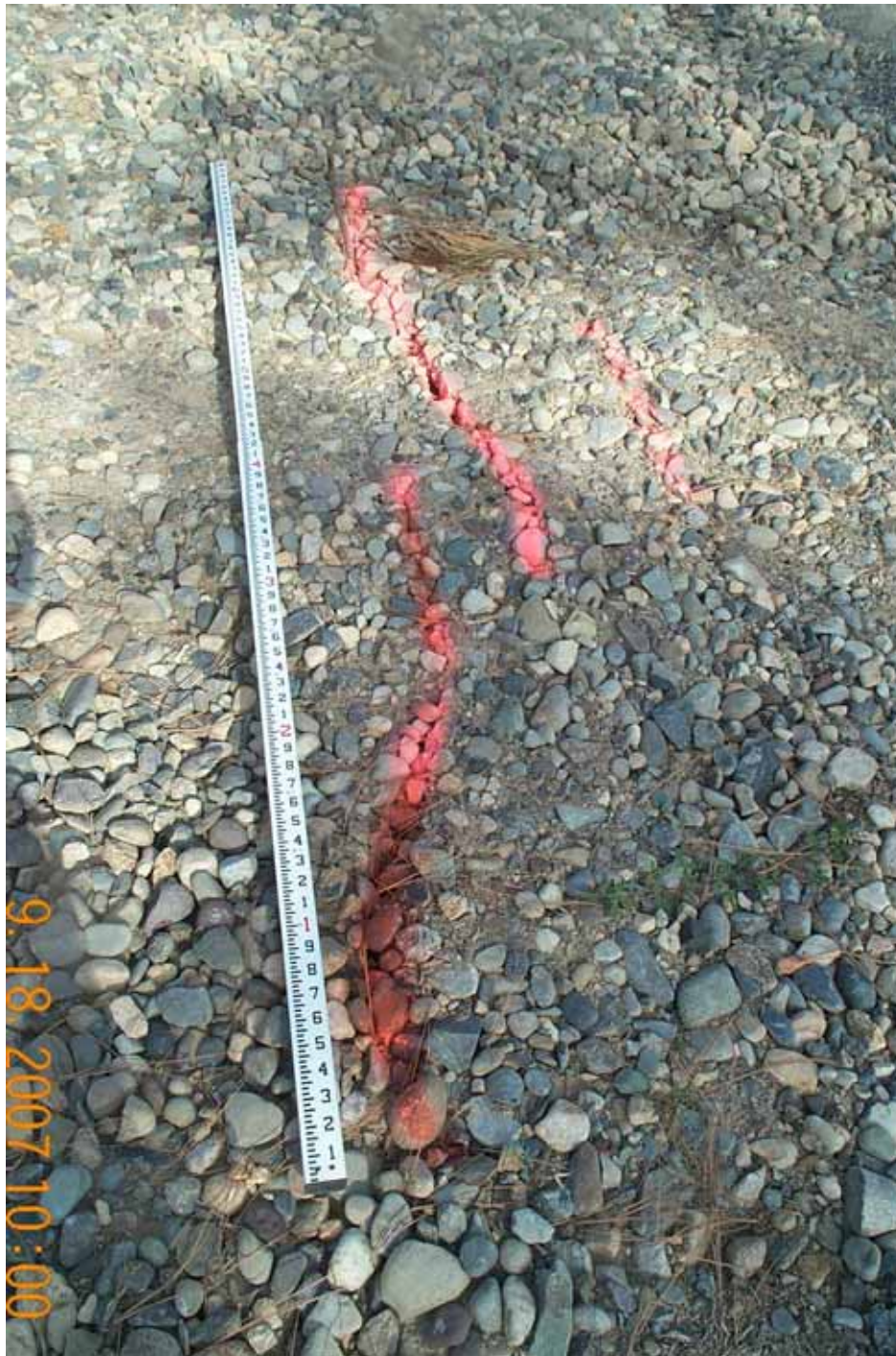
Photograph No. 2. View of to the north looking at extension cracks (orange paint) along the western side of the “slump” along the Fulton irrigation pipeline. Red dye was poured in the center crack prior to excavation. Fulton Dam, Methow Subbasin, Washington – Bureau of Reclamation Photograph by E. Lyon, September 18, 2007.
