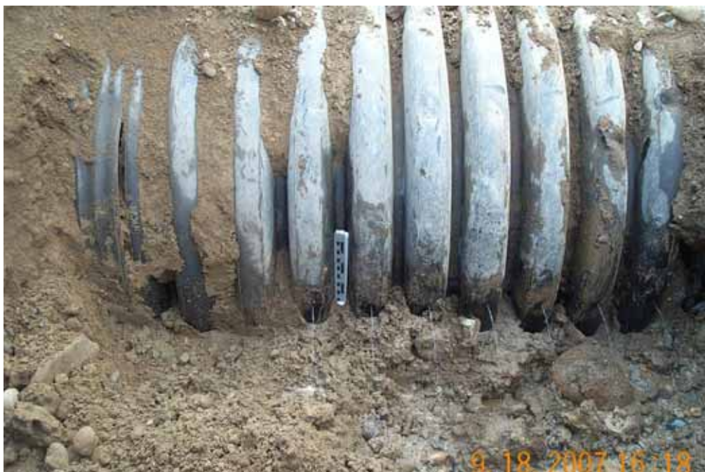
Photograph No. 7. View is to west looking at the Fulton irrigation pipeline exposed at depth. Note the horizontal alignment of the perforations leaking water along the pipe and the openness of the joint (left center in photograph). Fulton Dam, Methow Subbasin, Washington – Bureau of Reclamation Photograph by E. Lyon, September 18, 2007.
