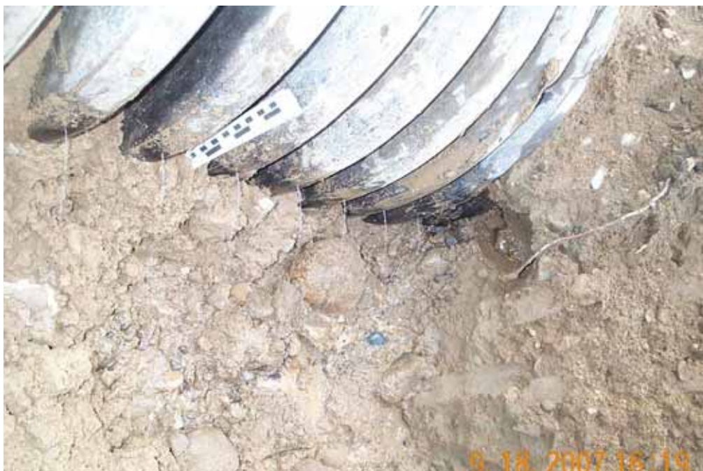
Photograph No. 8. View is to northwest looking at the perforations along the Fulton irrigation pipeline and the perforations leaking water. Fulton Dam, Methow Subbasin, Washington – Bureau of Reclamation Photograph by E. Lyon, September 18, 2007.
