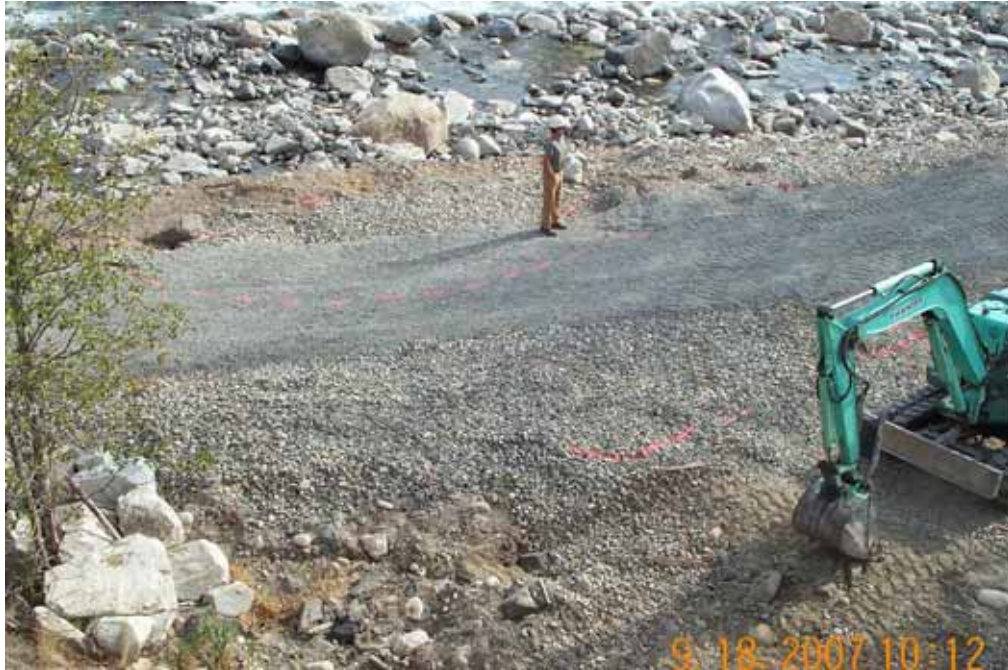
Photograph No. 5. View is to the east looking over the settlement area with extension cracks and slump marked by orange paint. Fulton Dam, Methow Subbasin, Washington – Bureau of Reclamation Photograph by E. Lyon, September 18, 2007.
