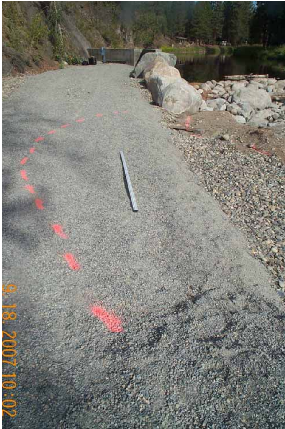
Photograph No. 3. View is to the north looking at the scarp (dashed orange paint) where the surface has settled about \pm 1 -foot along the Fulton irrigation pipeline. Fulton Dam, Methow Subbasin, Washington – Bureau of Reclamation Photograph by E. Lyon, September 18, 2007.
