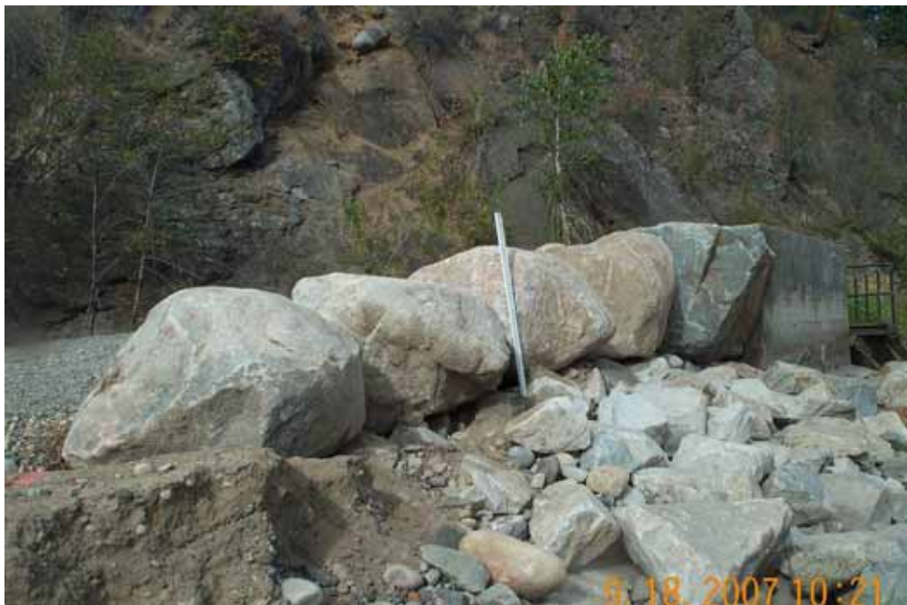
Photograph No. 16. View is to the west looking at scour that has occurred at the base of the 4-foot-diameter boulders placed on the right bank along the roughened channel. Three of the boulders are precariously held in place and are in jeopardy of toppling. Fulton Dam, Methow Subbasin, Washington – Bureau of Reclamation Photograph by E. Lyon, September 18, 2007.
