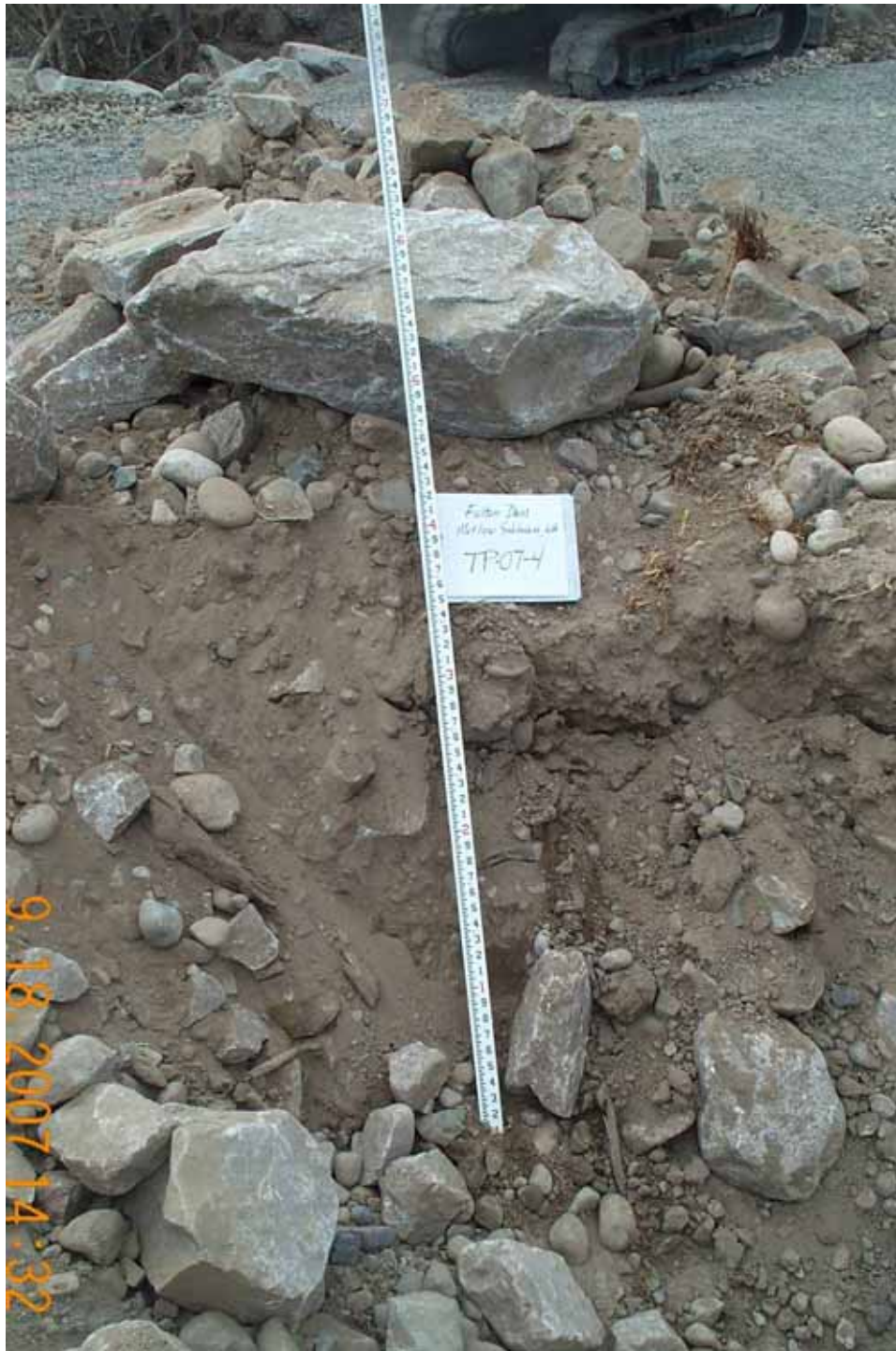
Photograph No. 14. View is to the north looking at test pit TP-07-4 excavated through the placed riprap along the roughened channel on river right. Fulton Dam, Methow Subbasin, Washington – Bureau of Reclamation Photograph by E. Lyon, September 18, 2007.
