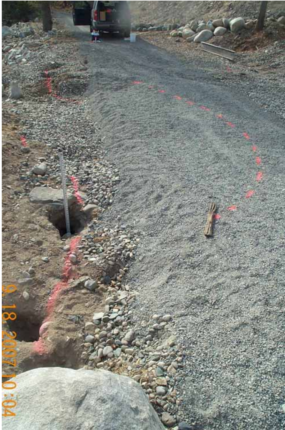
Photograph No. 4. View is to south looking at voids along the east side of the Fulton irrigation pipeline and the settlement area (orange paint). Fulton Dam, Methow Subbasin, Washington – Bureau of Reclamation Photograph by E. Lyon, September 18, 2007.
