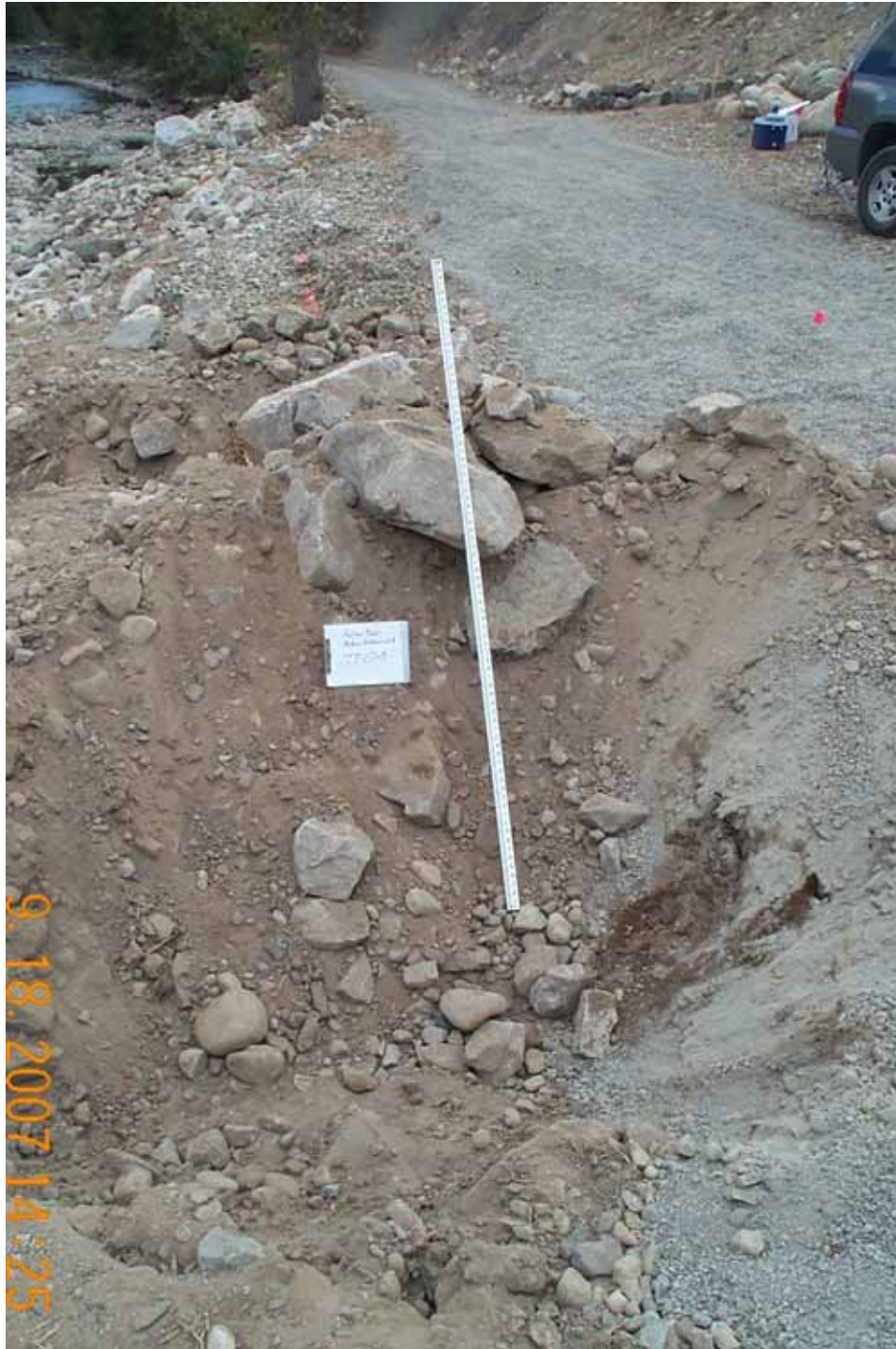
Photograph No. 13. View is to the south looking at test pit TP-07-3 excavated through the placed riprap along the roughened channel on river right. Fulton Dam, Methow Subbasin, Washington – Bureau of Reclamation Photograph by E. Lyon, September 18, 2007.
