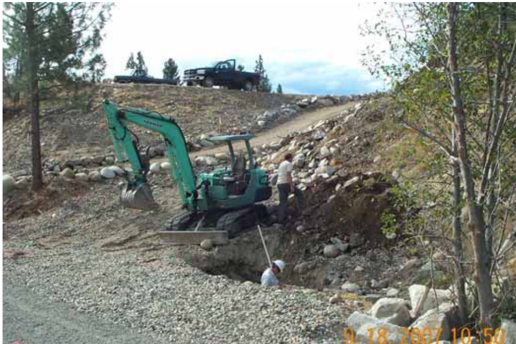
Photograph No. 10. View is to west looking at location of test pit TP-07-1 where a depression was filled with spoils along the Fulton irrigation pipeline. Fulton Dam, Methow Subbasin, Washington – Bureau of Reclamation Photograph by R. Link, September 18, 2007.
