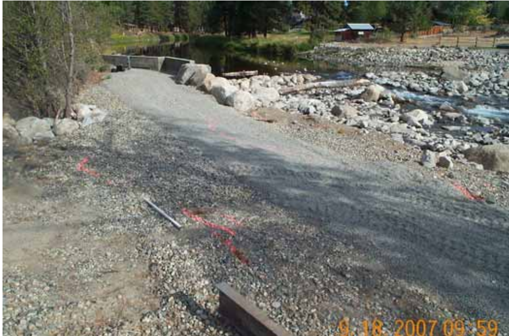
Photograph No. 1. View is to the north looking at extension cracks (orange paint) along the Fulton irrigation pipeline. Fulton Dam, Methow Subbasin, Washington – Bureau of Reclamation Photograph by E. Lyon, September 18, 2007.
