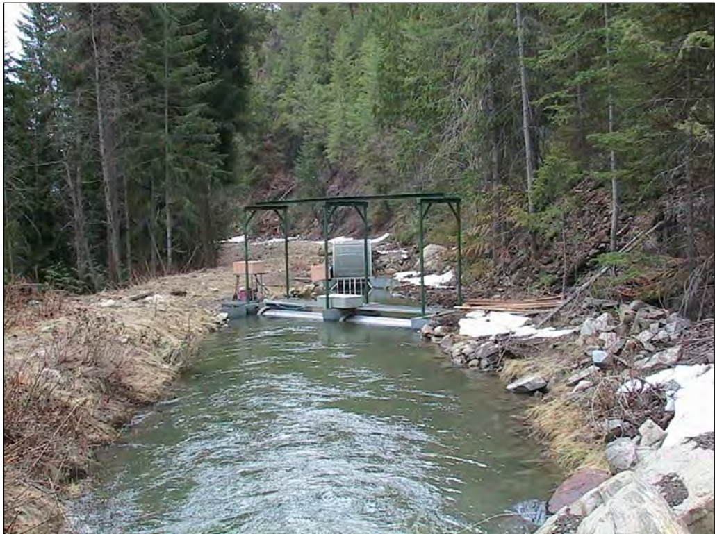
Photo A-2. Downstream view of the fish screen, staging area, and pipe bench prior to construction. The canal and fish screen are running near capacity which is about 13 cfs.
