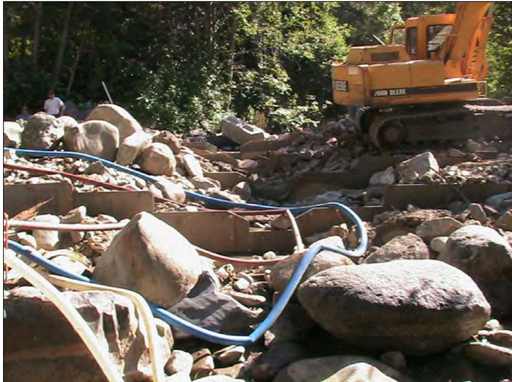
Photo A-12. Upstream view of all four weirs set in place and backfilled. Large rocks are being randomly placed to act as roughness to the flow and aid in fish passage at various flows. The staggering of the low-flow notches is noticeable.
