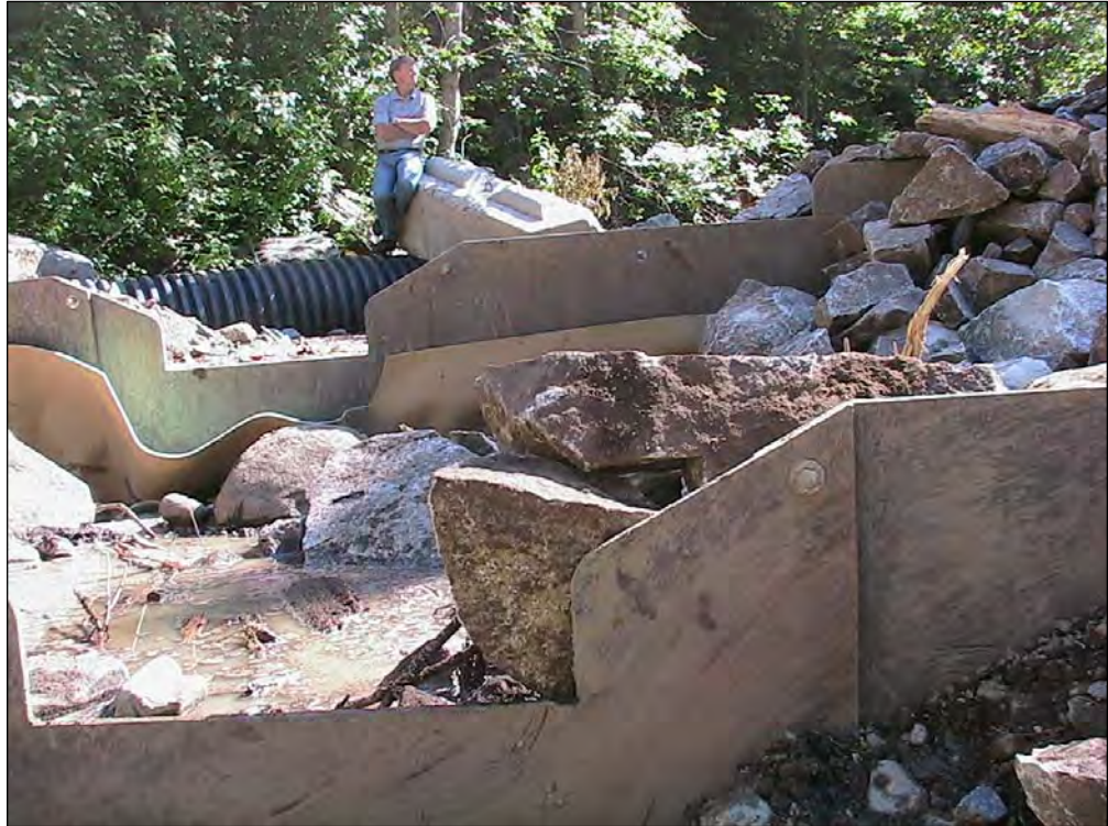
Photo A-13. Upstream view of the low-flow notches after placement of some of the larger rocks designed to interrupt and roughen the flow creating lines and eddies to increase fish passage opportunities.
