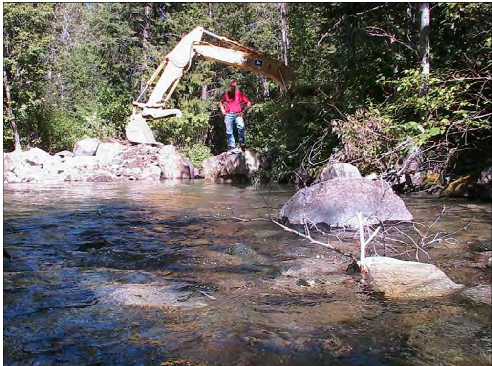
Photo A-14. A view looking downstream toward the entrance to the ditch. A large rock was placed on the creek bank upstream of the ditch entrance to block debris and logs from being forced into the ditch by the current.
