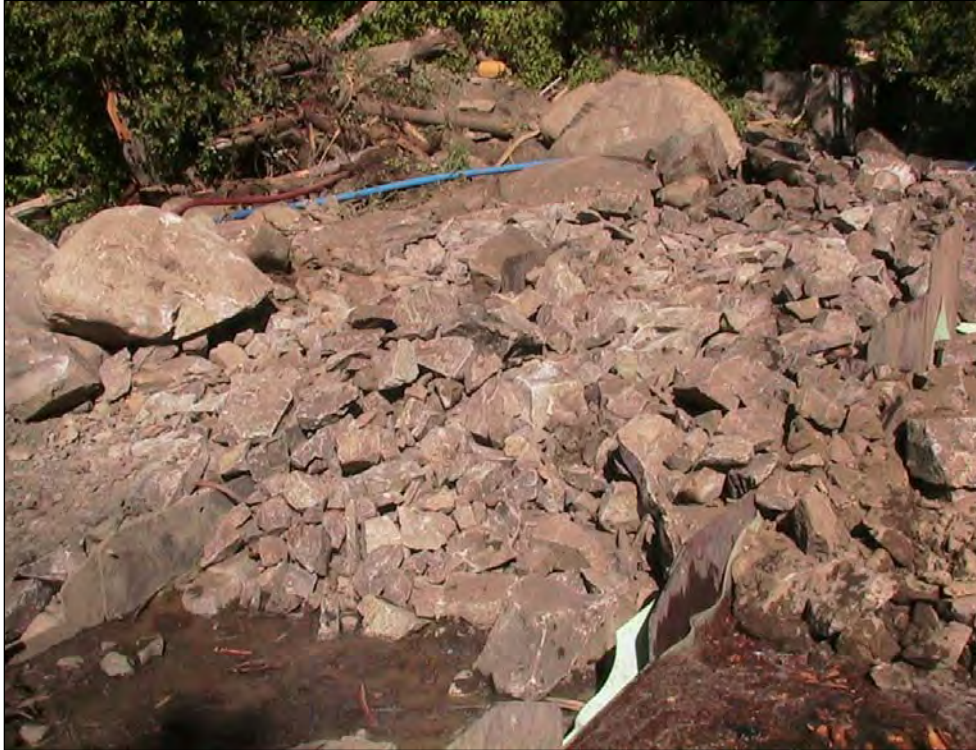
Photo A-11. View of the backfilled weirs: final grading and final fill were completed with talus material. To aid in fish passage, several large-diameter rocks (at left) were randomly placed to help break up the flow, reduce water velocity, and add pockets of slow-moving water.
