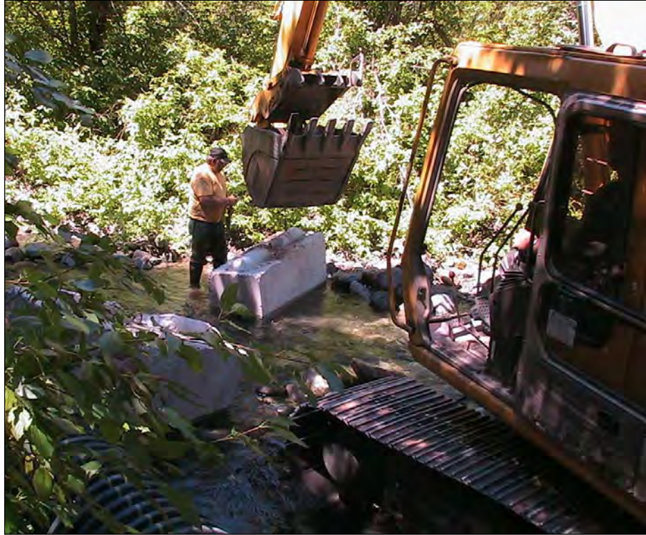
Photo A-3. Construction begins with placement of ecology blocks for the cofferdam about 25 feet upstream of the existing structure. The ecology blocks divert the creek flow in a 30-inch diameter HDPE pipe which transports the water to the headworks.
