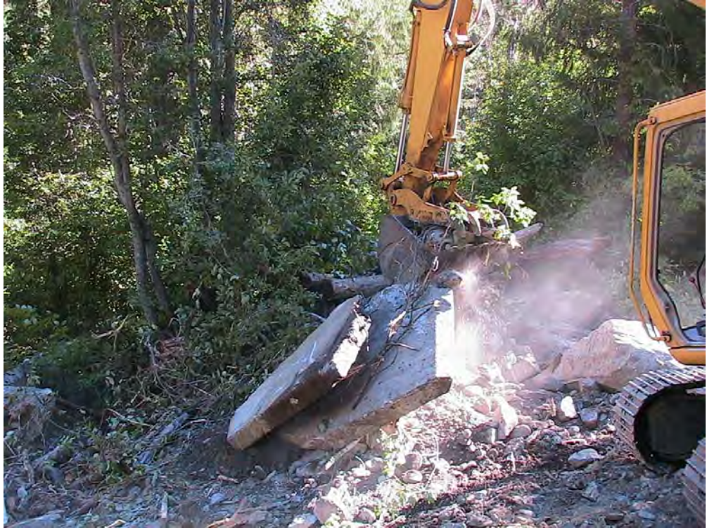
Photo A-5. The excavator breaks up a section of the previous concrete diversion channel which had been washed out in the 1948 flood.
