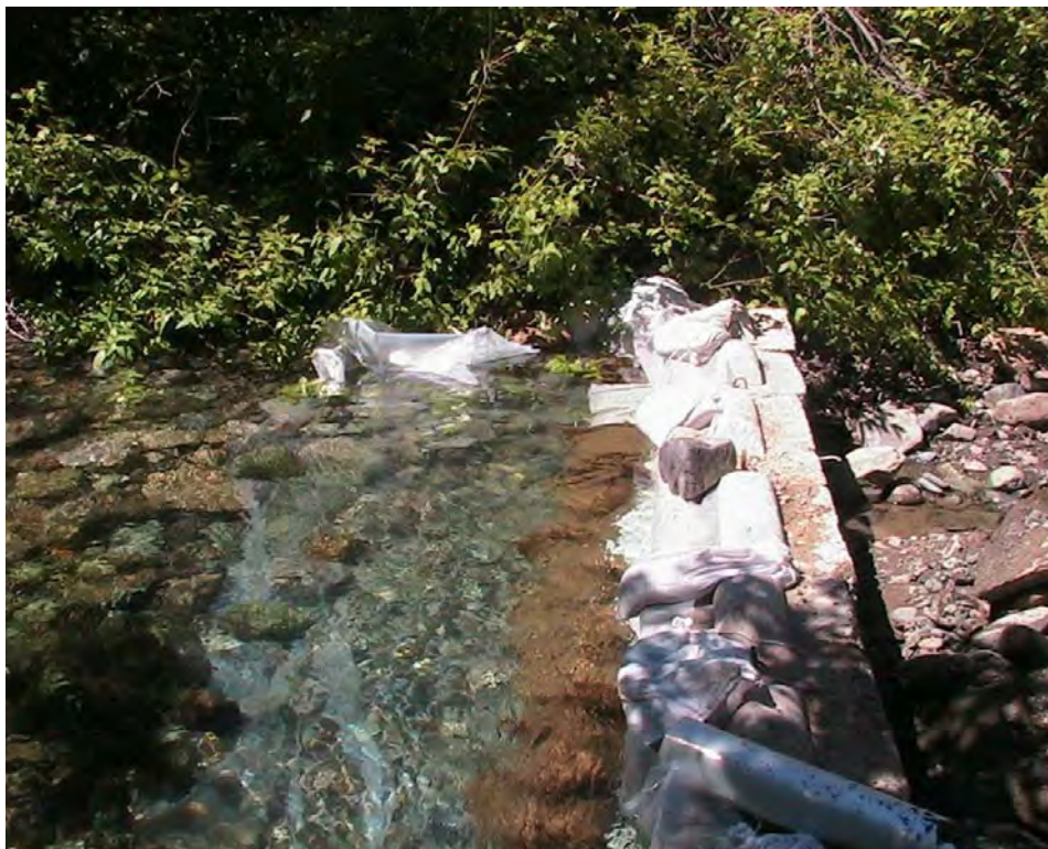
Photo A-4. Completed cofferdam including sandbags and plastic. The creek is diverted into a pipe just out of the bottom of the photo. Dewatered channel can be seen at the right of the photo.
