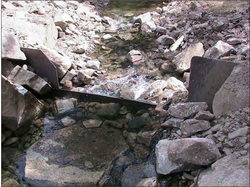
Photo A-1. View of steel weir at the entrance to the ditch about 60 feet upstream of the intake structure. The weir is designed to provide grade control and prevent cutting of the canal section during high flows.
