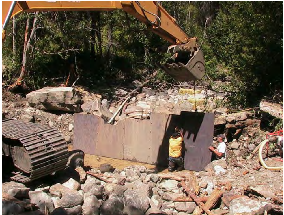
Photo A-6. Assembling the downstream weir (#4) first. It was critical that the middle three plates (of ten) be level and at the proper elevation, so they were bolted together on the bank and set first. Average completion time for each weir was one day.
