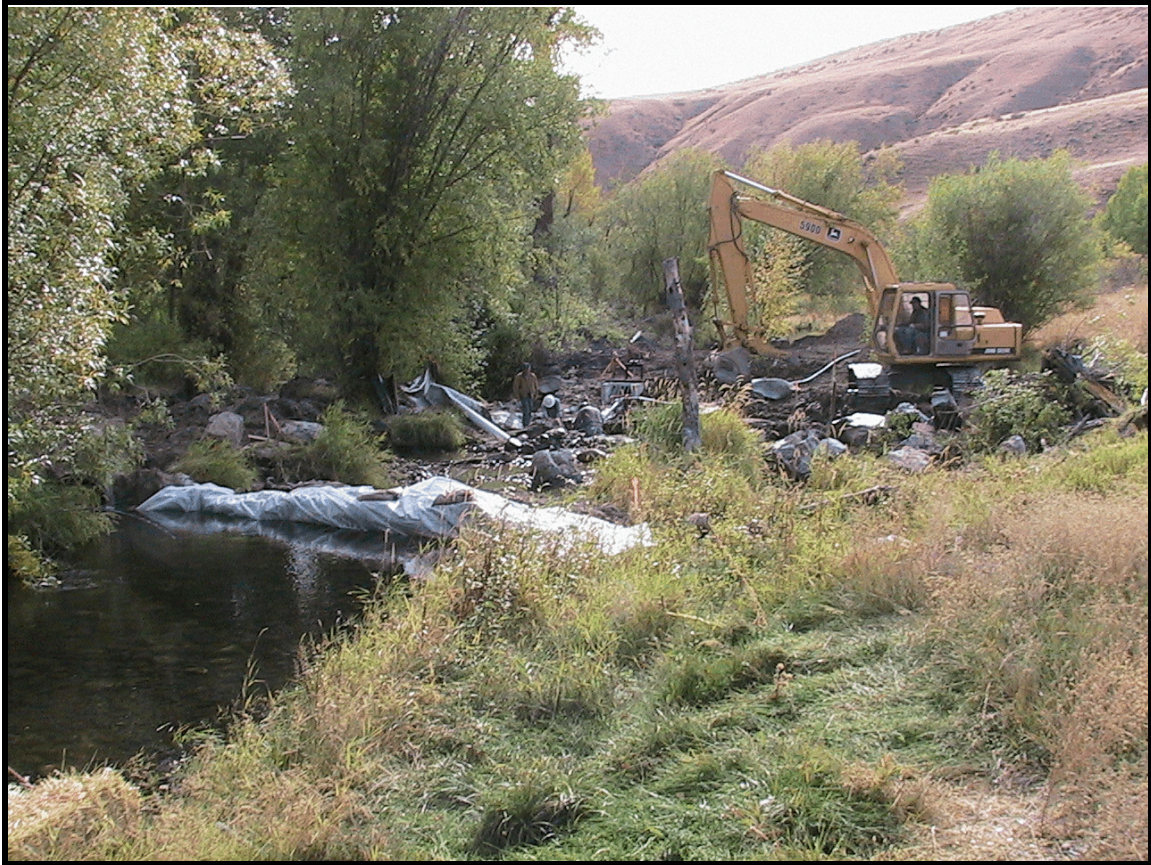
Photo A-25. The Upper Stokes project job site during construction. The cofferdam is at left center.
