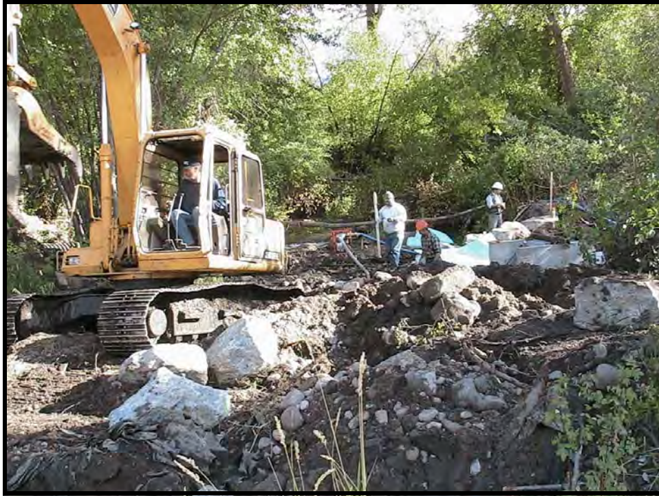
Photo A-9. Looking downstream, the new diversion structure (at middle right) has been set.
