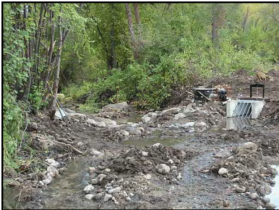
Photo A-10. Looking downstream at Weir No. 1, which has been lined with geotextile and then backfilled. The pipe trench has also been backfilled.
