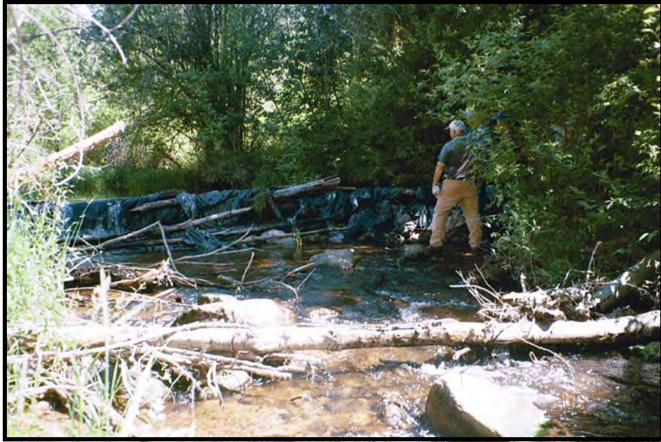
Photo A-1. Looking upstream at original Upper Stokes Diversion Dam (photo taken July 2002).
