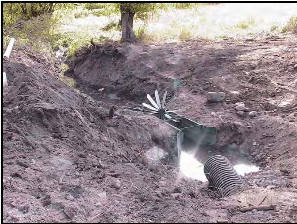
Photo A-16. The diversion pipe extension and the ditch transition at the fish screen. Note the benching of the ditch slopes.
