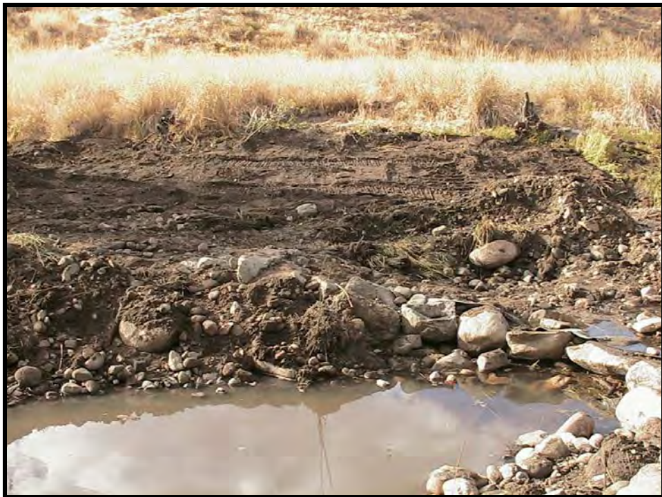
Photo A-18. Looking upstream at Weir No. 2 and the rebuilt stream bank.
