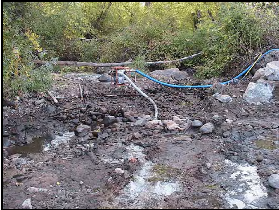
Photo A-3. Looking downstream at the double-drop Weir No. 1; rock has been placed and tied into the right bank. This is the upper portion of the A-shaped weir. The suction pump in center picture is sending seepage water into the woods.
