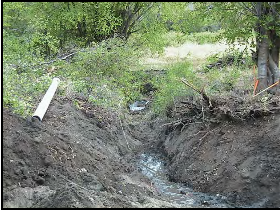
Photo A-13. Along the diversion ditch, just downstream from the fish screen. The new ramp flume is shown near the center of the picture. This portion of the ditch have been cleared of vegetation and deepened.
