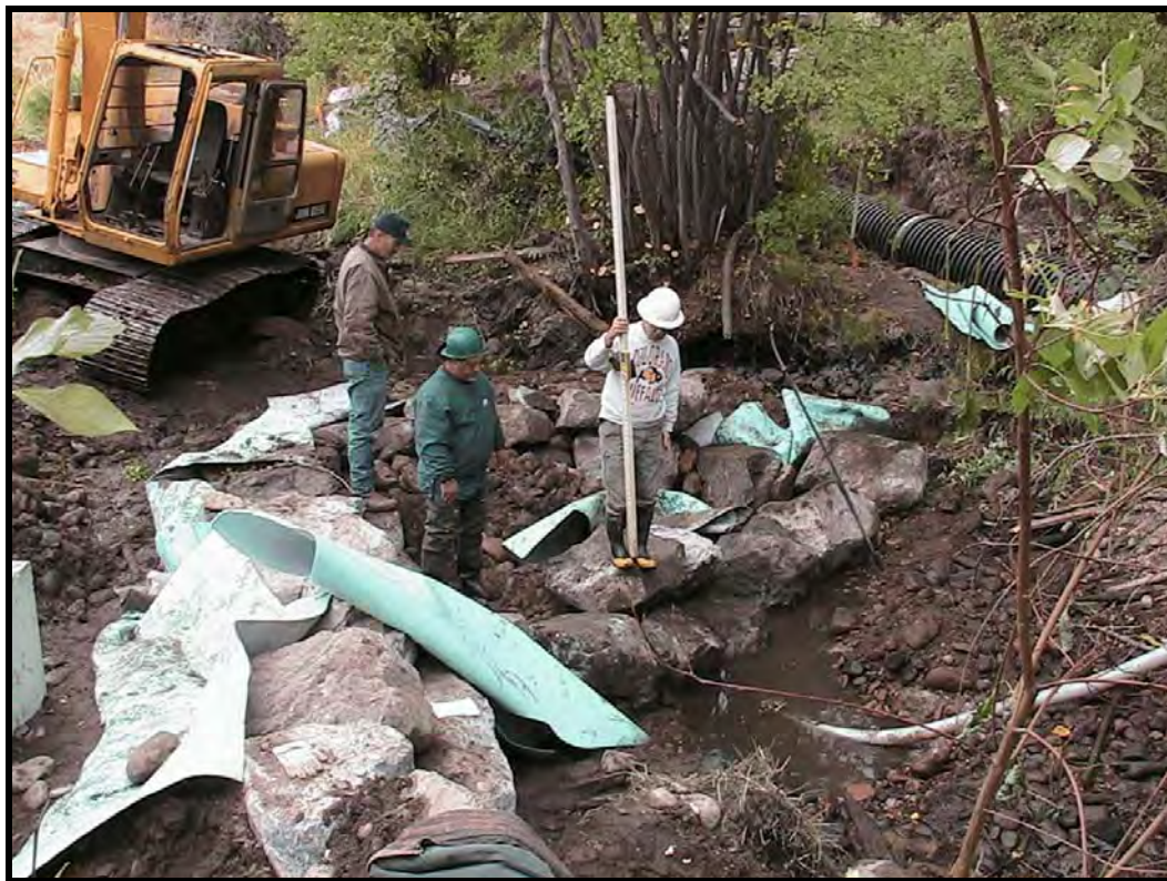
Photo A-6. Looking upstream at Weir No. 1. A section of the dewatering pipe can be seen at the upper right; the seepage-pump line is at lower right; and the new diversion box is at the lower left.
