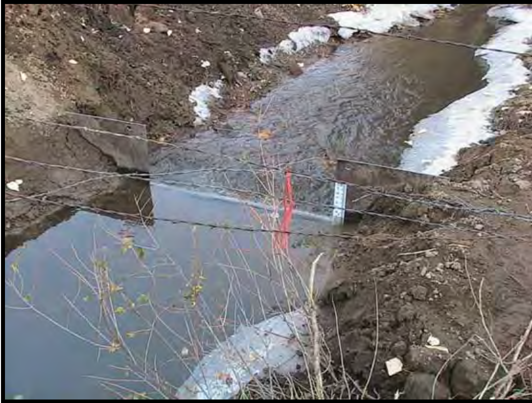
Photo A-23. Installed by Okanogan Conservation District, this new, sharp-crested rectangular measuring weir is located on the irrigation ditch about 400 feet downstream of the diversion point.
