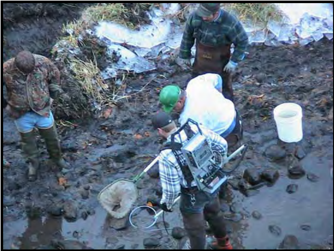
Photo A-9. USFS and Okanogan Conservation District staff electroshocking fish in construction area for release downstream.
