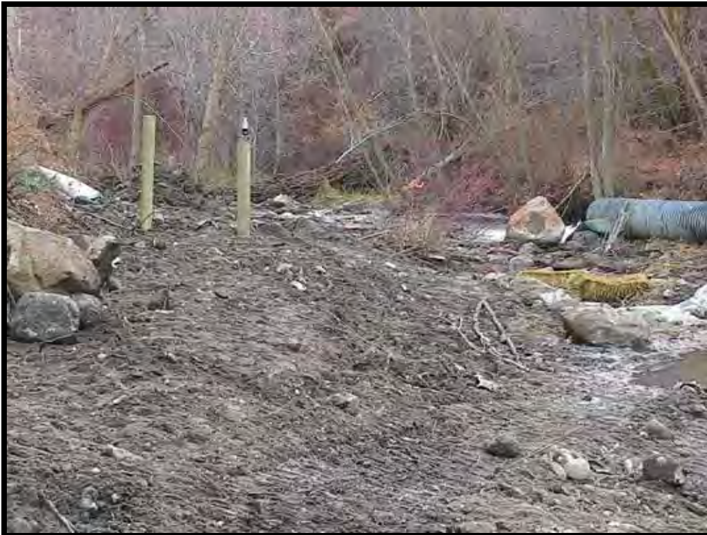
Photo A-24. Looking downstream from left side, the majority of construction is complete, and the temporary dewatering pipe is still in place. Site rehabilitation is underway; the diversion pipe ends just beyond the new fence posts.
