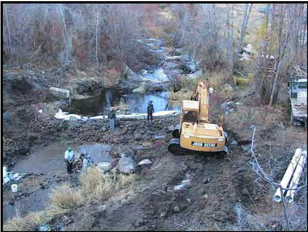
Photo A-8. Ecology-block-and-plastic cofferdam in place. Temporary irrigation pipe has been backfilled. Staff from WDFW are electroshocking fish.
