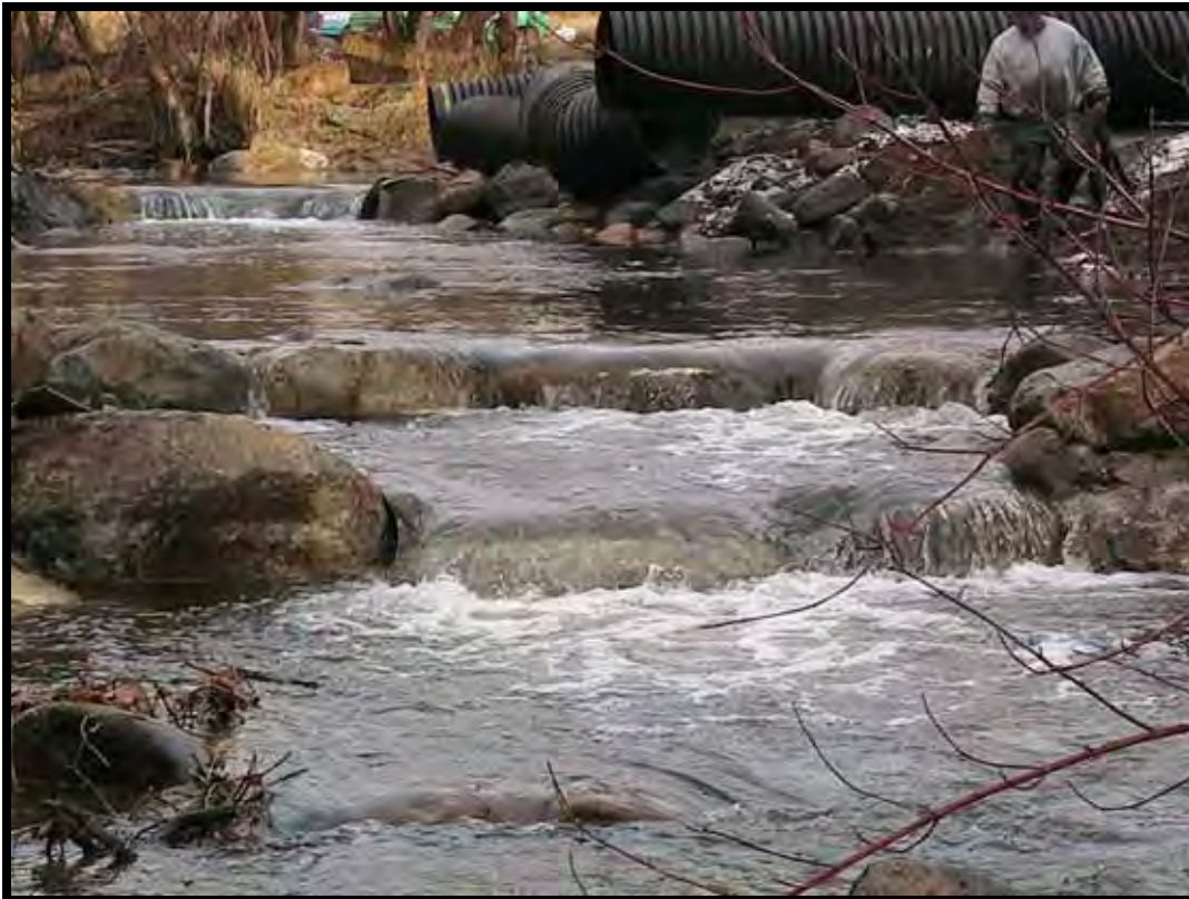
Photo A-28. Closer upstream view of project. Weir No. 2 is in the foreground and Weir No. 1 in the background. Flows are normal for the time of the season, about 6 cfs.
