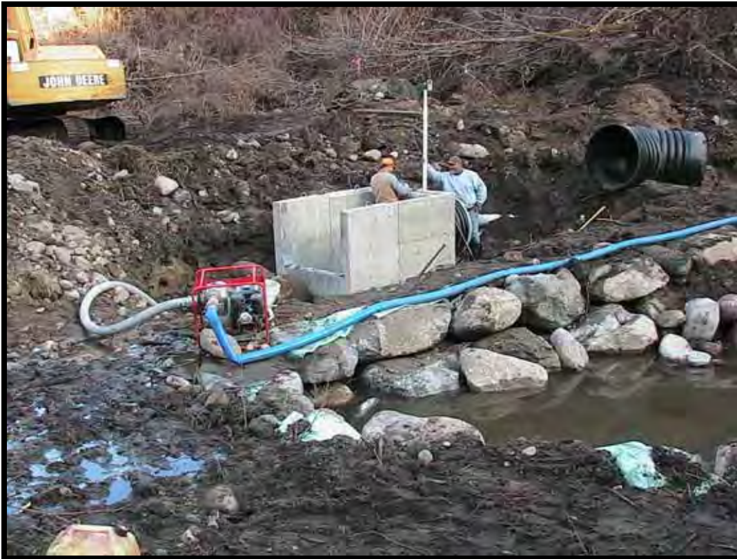
Photo A-17. Setting concrete control structure on right side of V-type Weir No. 1. Pump with blue pipeline is removing seepage water.
