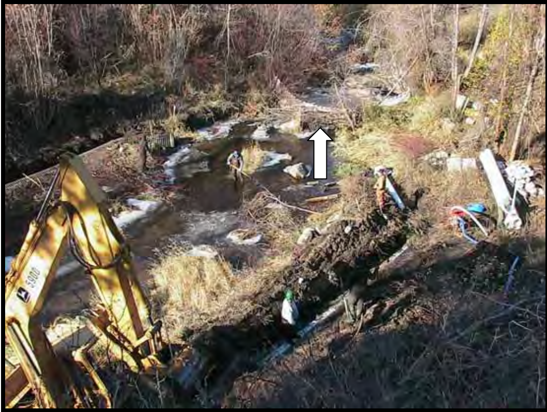
Photo A-7. Dewatering pipe in place (upper left); crew placing temporary irrigation pipe (lower right). Note fish-blocking net across stream (arrow). The cofferdam was built where the worker in the creek is standing.
