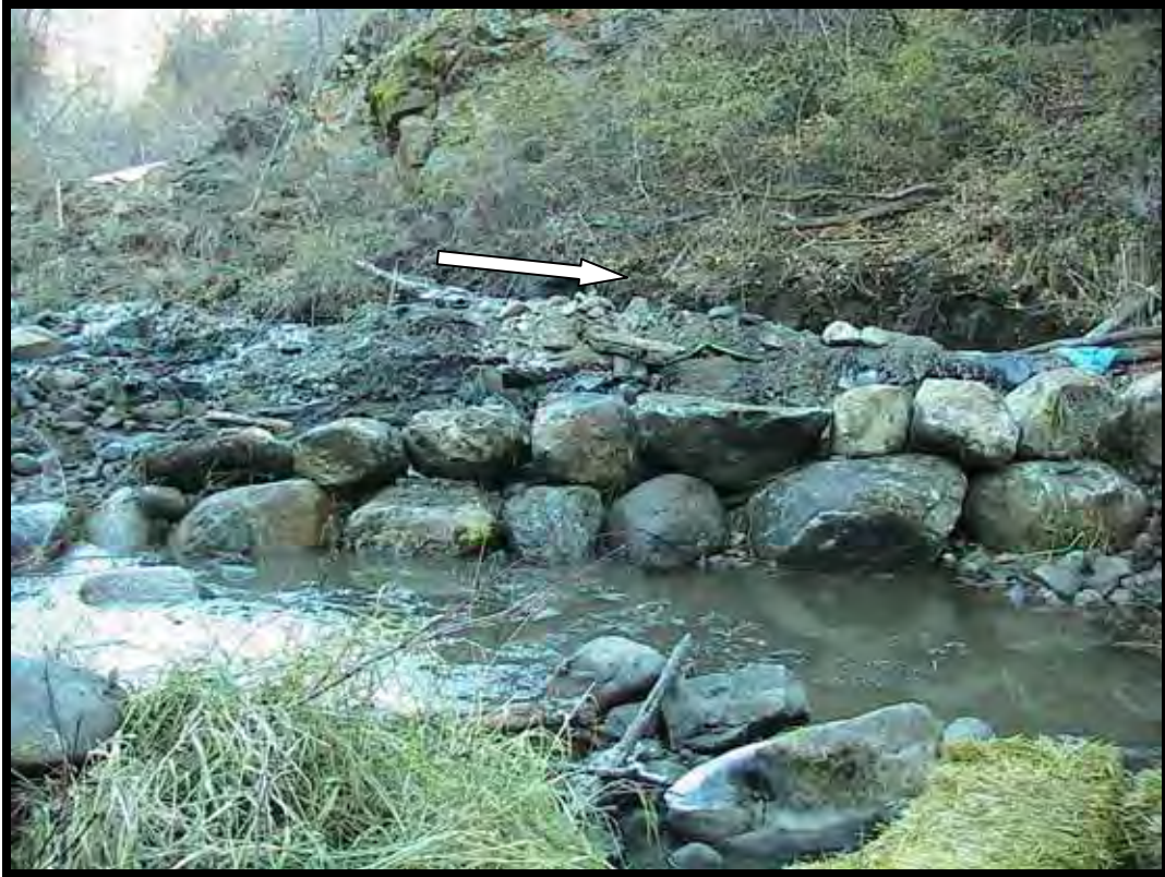
Photo A-11. Looking upstream at right arm of A-type Weir No. 2. The direction of flow of the temporary irrigation pipeline is indicated by the arrow. The cofferdam is out of view around the corner (upper left).
