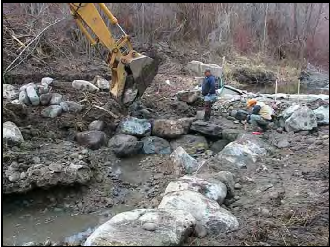
Photo A-12. Looking upstream at left arm of V-type Weir No. 1 under construction.
