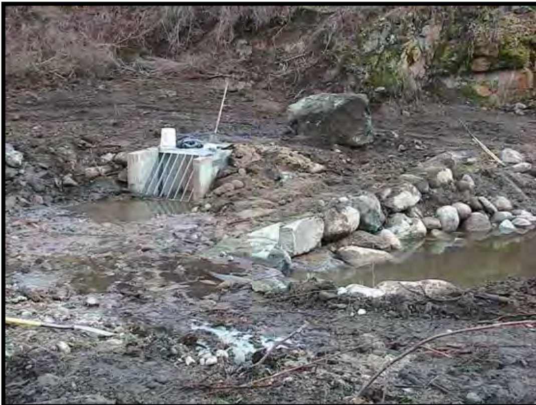
Photo A-18. On left side upstream from A-type Weir No. 2, concrete diversion structure with trashrack in place. The permanent diversion pipe is in place and backfilled. Note the metal strap holding the two sidepieces of the trashrack. In all, six straps were used.
