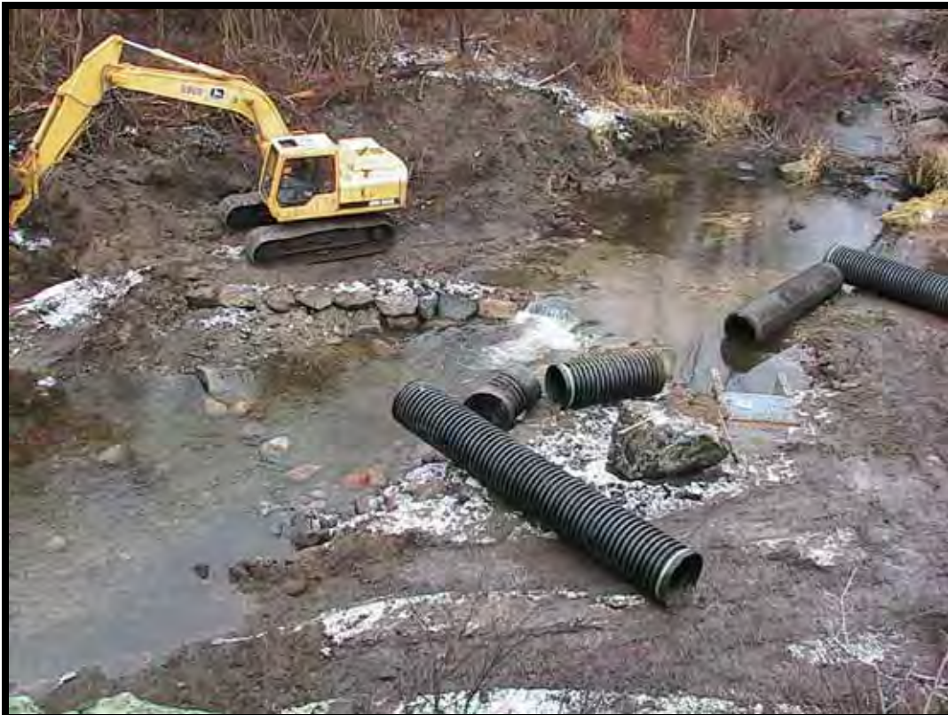
Photo A-26. Looking downward at Weir No. 2; the dewatering pipe has been removed and has been temporarily set along the stream. The excavator is finishing the rock weir.
