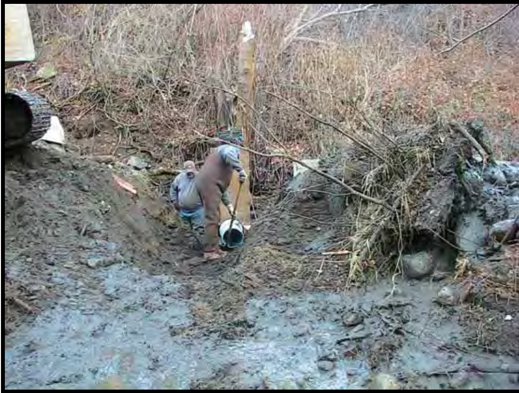
Photo A-21. Contractor installing sluice gate in diversion ditch just upstream of turnout structure.
