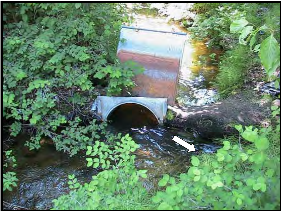
Photo A-4. Looking downstream at the original ditch headgate; the arrow indicates the direction of flow of the wasteway ditch. The former headgate was located about 50 feet downstream from the diversion dam. (September 2003)
