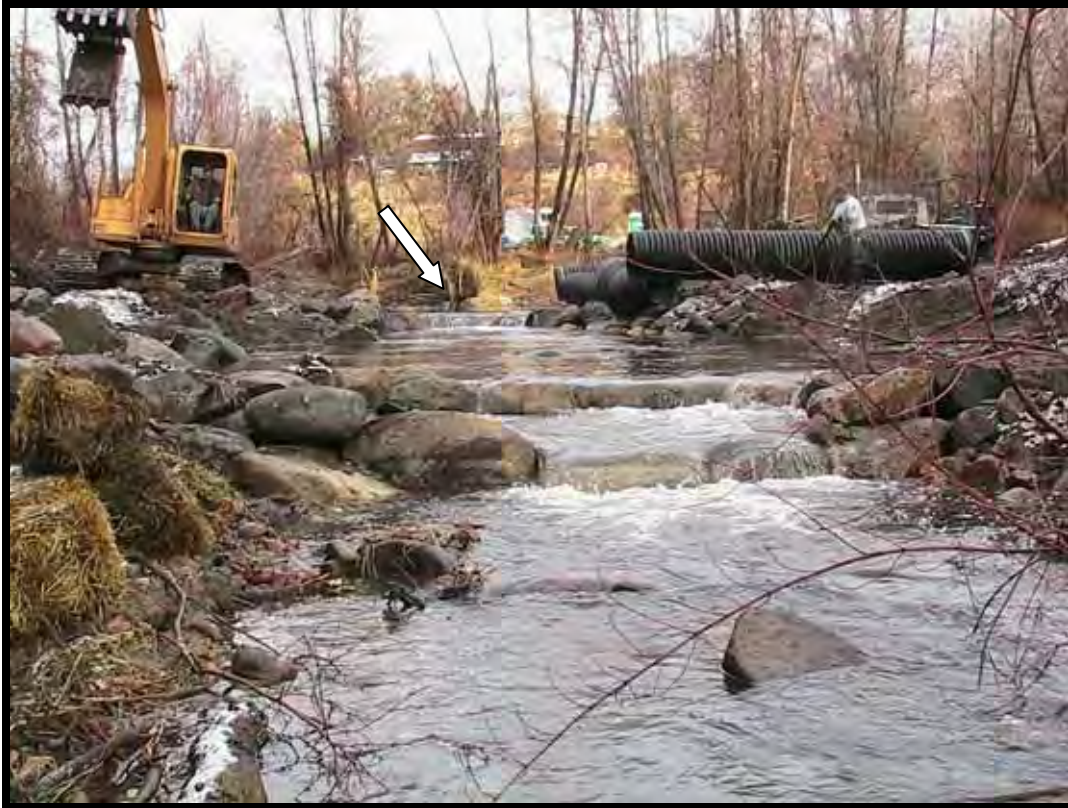
Photo A-27. Looking upstream at completed weirs. The A-type Weir No. 2 and the V-type Weir No. 1 is indicated by arrow. The dewatering pipe is soon to be moved offsite.
