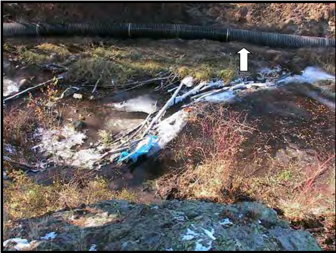
Photo A-3. Looking down at original diversion dam; the original ditch is in lower left of photo. The contractor-installed dewatering pipe is indicated by arrow.
