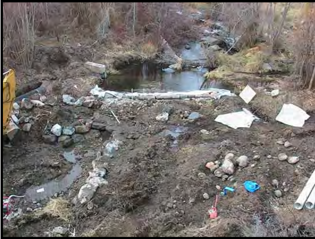
Photo A-15. Looking at site of V-type Weir No. 1 just downstream from cofferdam; contractor working on left side.
