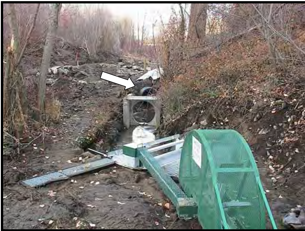
Photo A-20. View looking up diversion ditch; the new fishscreen is in place. Behind the turnout structure (arrow) is the end of the 30-inch-diameter permanent diversion pipe.
