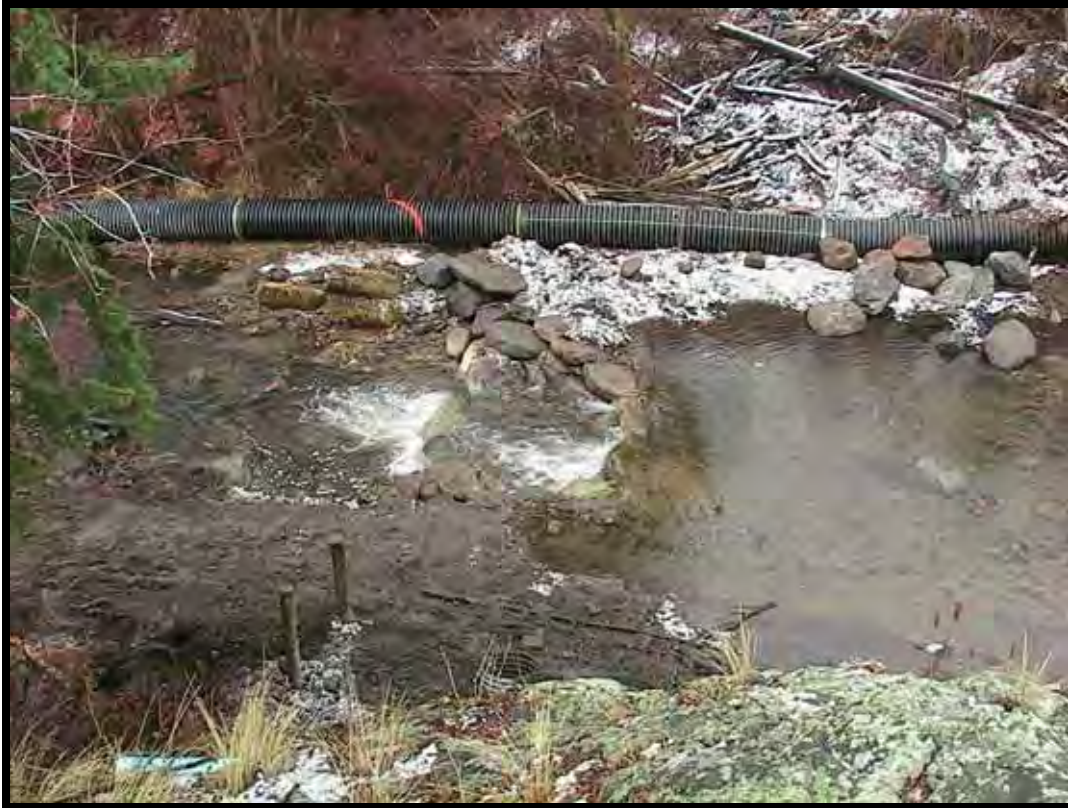
Photo A-25. Looking downward at completed A-type Weir No. 2. The cofferdam has been removed and normal seasonal flows are in the stream channel.
