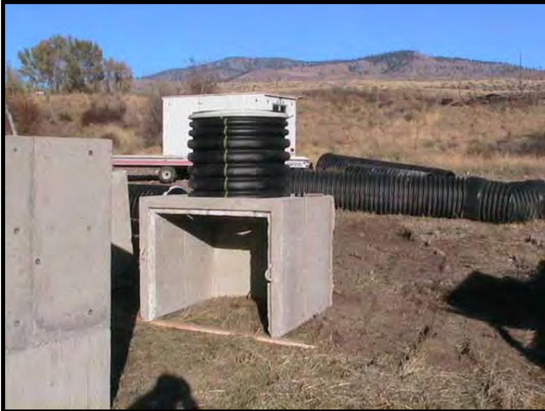
Photo A-16. Viewing back section of new diversion control box; the new turnout structure is at the left side of photo.
