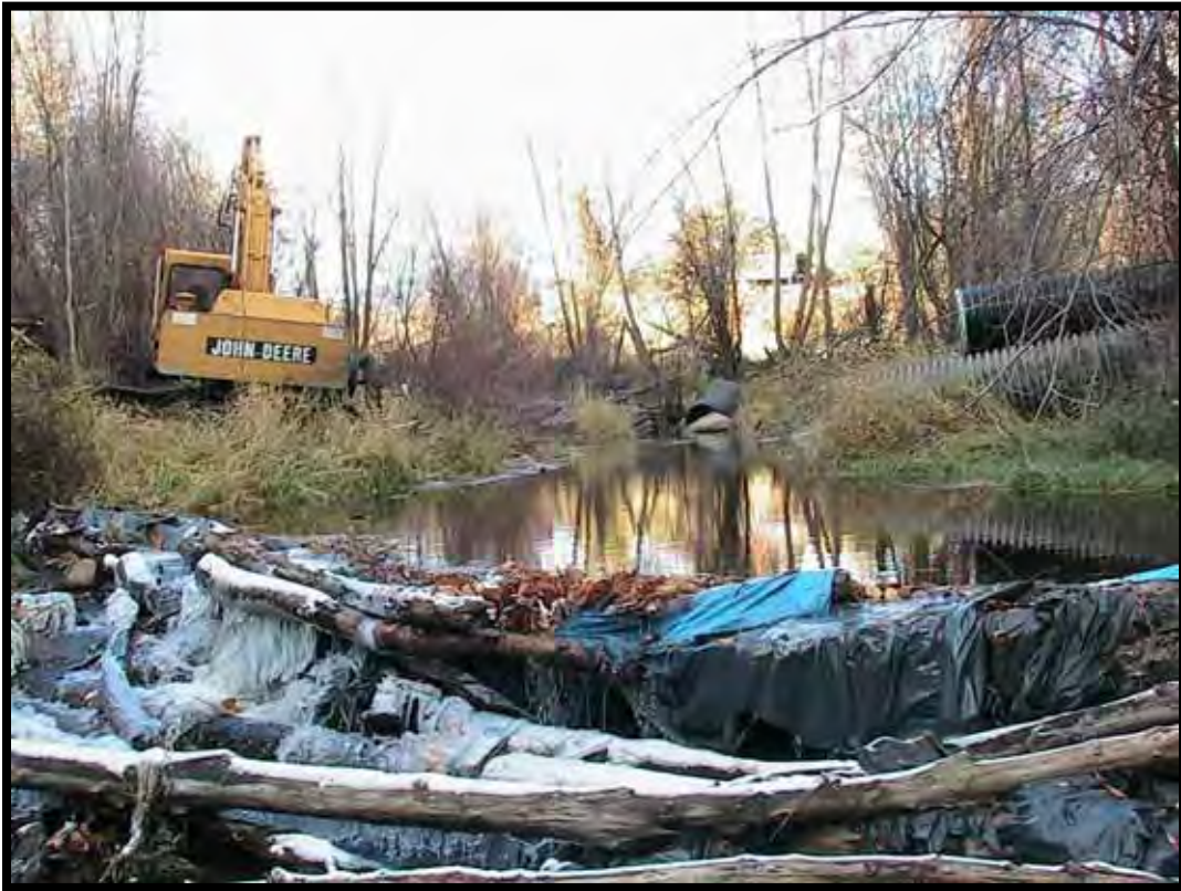
Photo A-6. The dewatering pipe just prior to installation; the pipe was to be installed on the right side of the creek, where the excavator is sitting.
