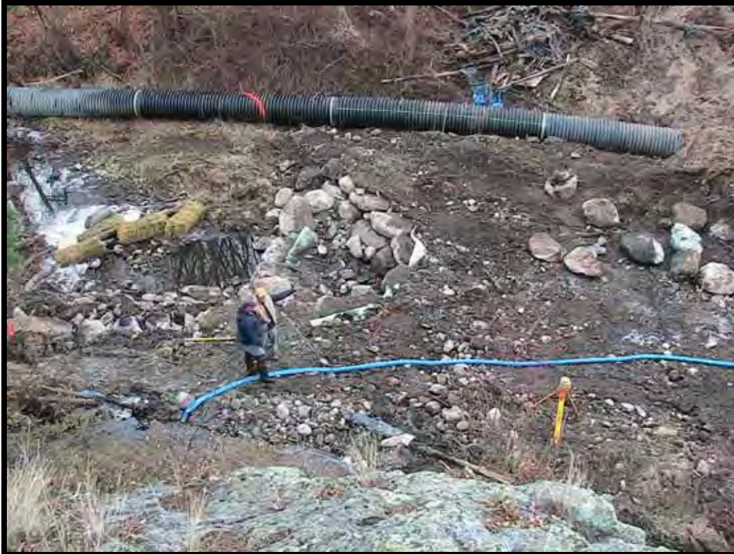
Photo A-14. Looking down at nearly completed Weir No. 2. The left arm of the weir will extend to the orange paint-mark on the pipe.
