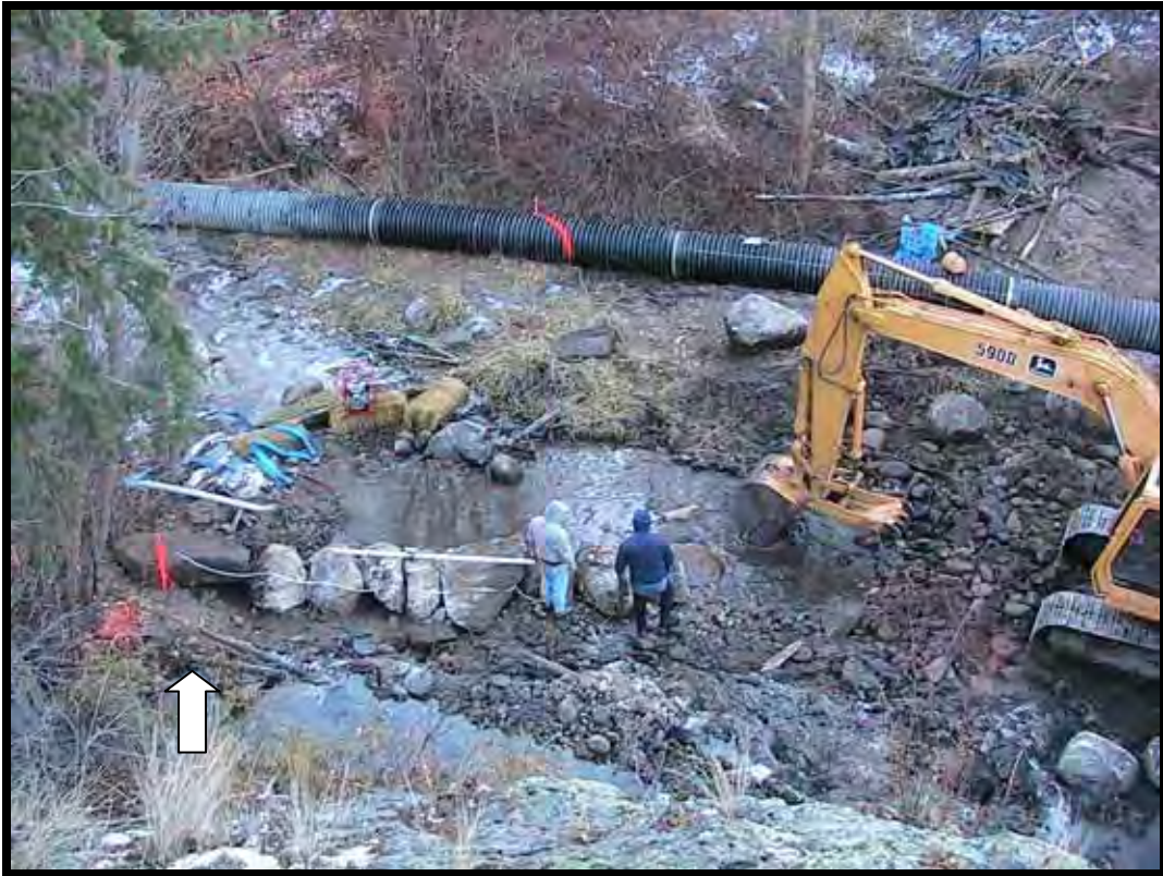
Photo A-10. Contractor constructing Weir No. 2, a double-drop A-type. Irrigation water is being supplied by temporary diversion pipeline (arrow).
