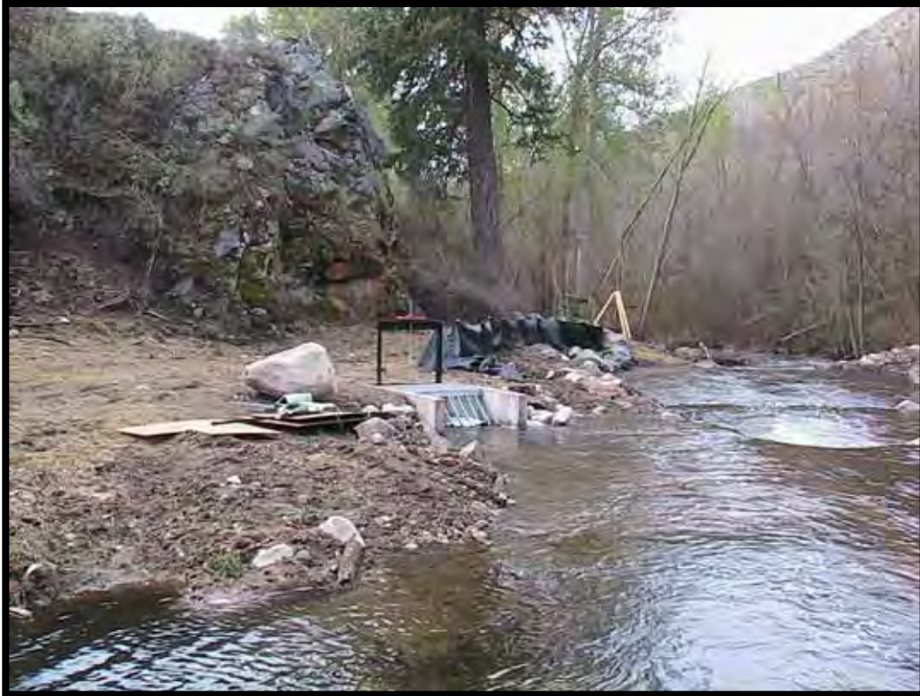
Photo A-29. Looking downstream at the new diversion box; Weir No. 1 is creating the vortex in the middle-left of the photo. (April 2004)
