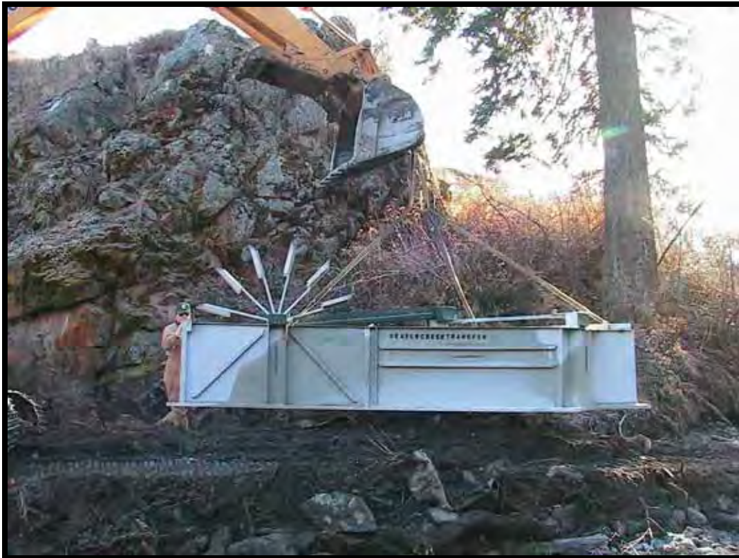
Photo A-19. Track hoe moving new fishscreen structure for placement in diversion ditch.
