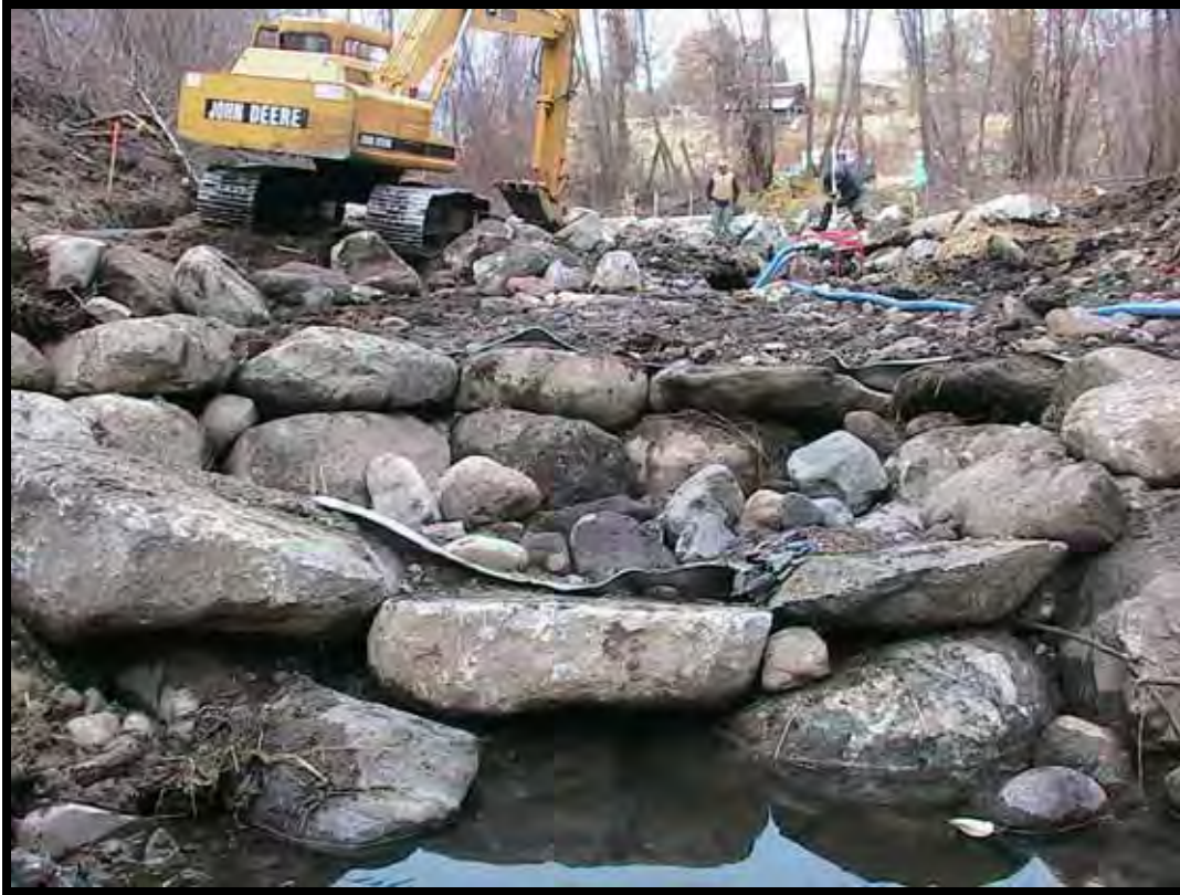
Photo A-13. Looking upstream at completed A-type Weir No. 2. Track hoe is working on upstream No. 1 “V” weir.
