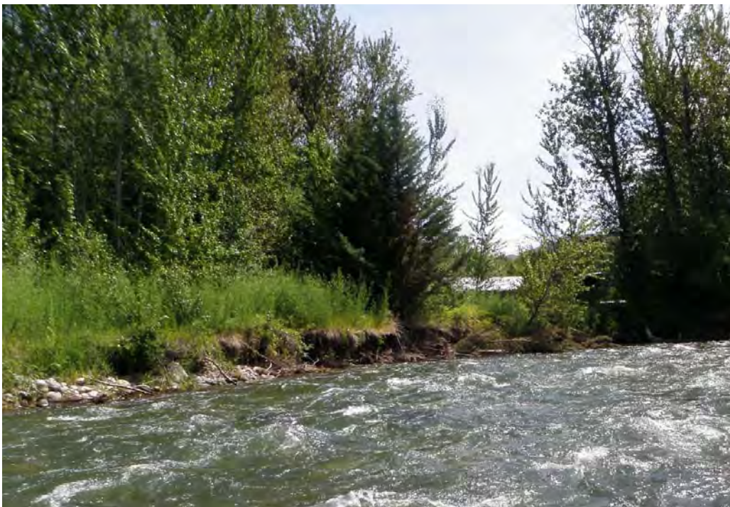
Figure 16. View of the bank erosion on the left bank near RM 5.0.
