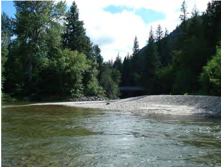
Photograph No. 10. View is to the south looking downstream at riprap placed along river left. (Subreach PR-IZ-4 – RM 21.2 – Reclamation photograph by R. McAfee, 2008).
