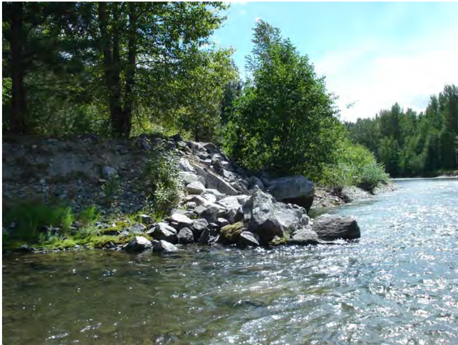
Photograph No. 20. View is to the south looking downstream at erosion along the upper extent of a levee along river left. Preston Reach – Entiat Subbasin, Washington – Bureau of Reclamation Photograph by R. McAfee August 21, 2008.
