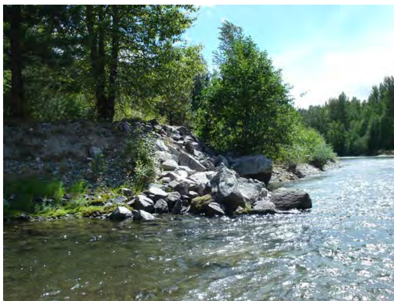
Photograph No. 5. View is to the south looking downstream along river left at the upstream end of a levee that is starting to fail. (Subreach PR-DOZ-5 – RM 22.3 – Reclamation photograph by R. McAfee, 2008).
