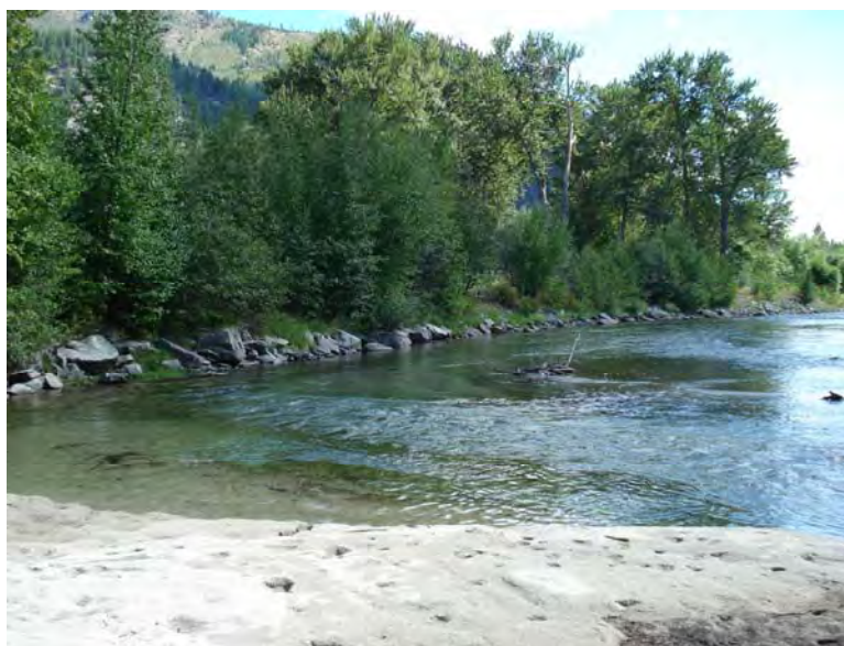
Photograph No. 7. View is to the south looking downstream at riprap placed along a levee on river left. (Subreach PR-DIZ-3 – RM 21.9 – Reclamation photograph by R. McAfee, 2008).
