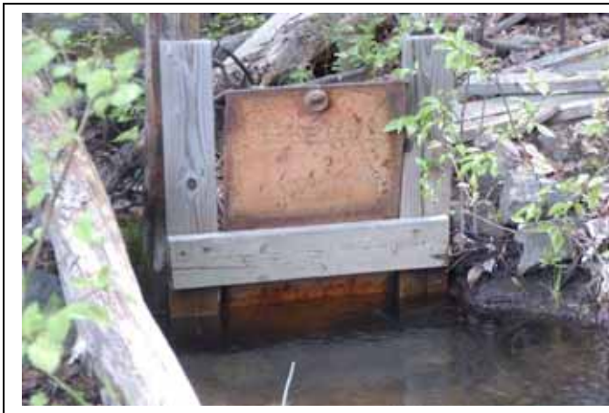
Existing non-functional Headgate
