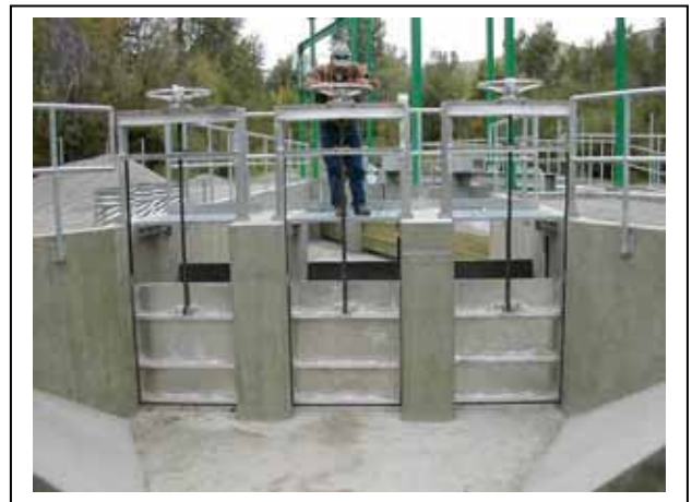
MVID West Screens
