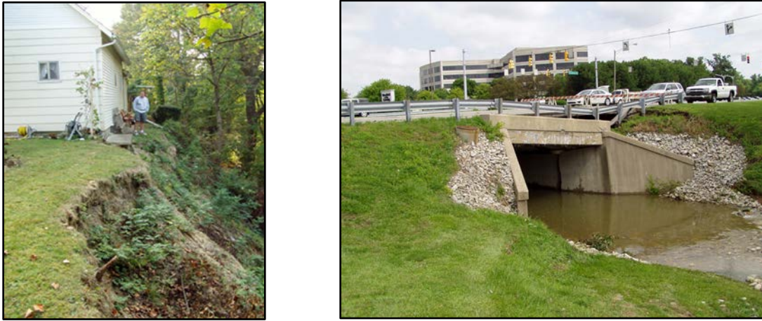
Figure 6. Examples of impacts of fluvial-erosion hazards in Indiana include the threat of loss or major damage to a residence (left) and damage to a heavily travelled urban bridge in Indianapolis (right).
