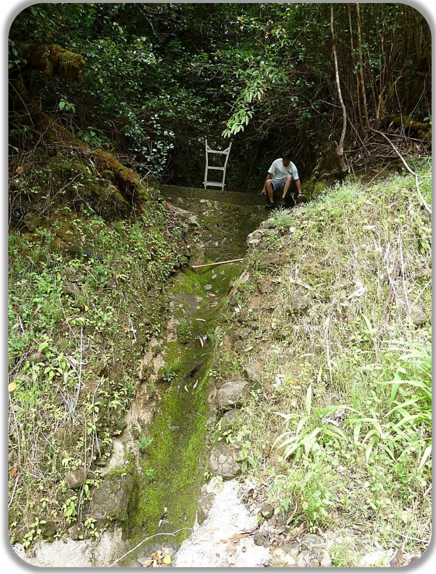
New Hamakua Ditch, a short opening
