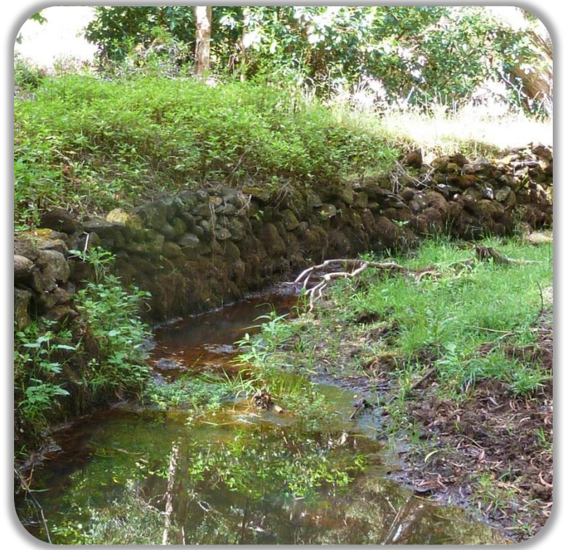
Spreckels Ditch, earthen material on right wall and stacked rocks on left wall
