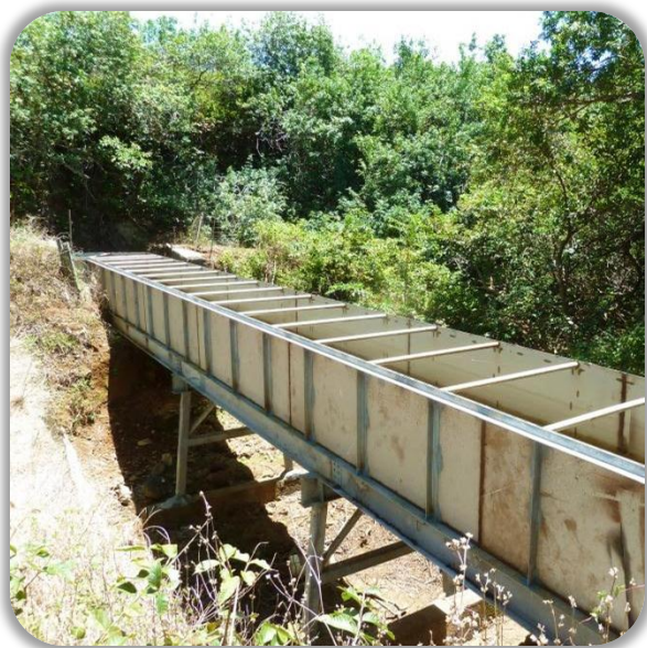
Lowrie Ditch, stainless-steel flume
