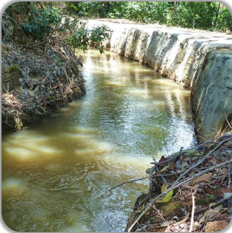
Lowrie Ditch, concrete on right wall (repaired) and earthen material on left wall
