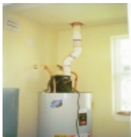
Power vented hot water heater
