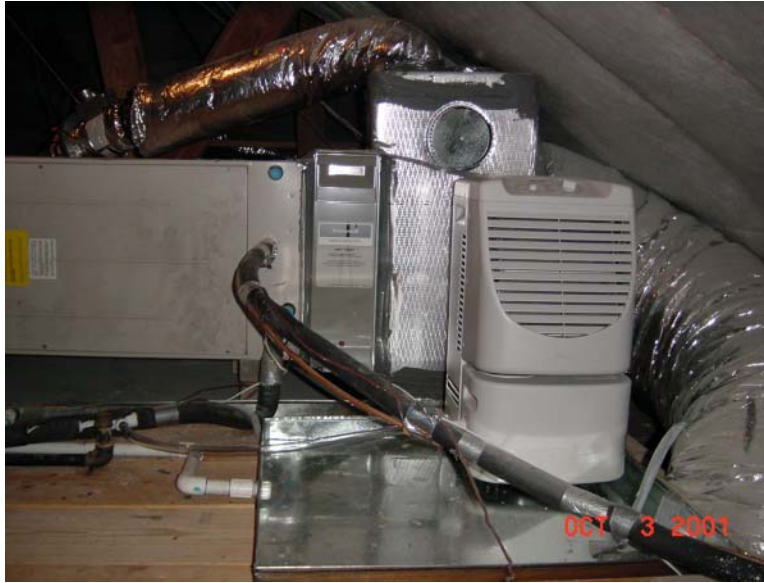
Figure A-2a. Stand-alone dehumidifier in conditioned attic
