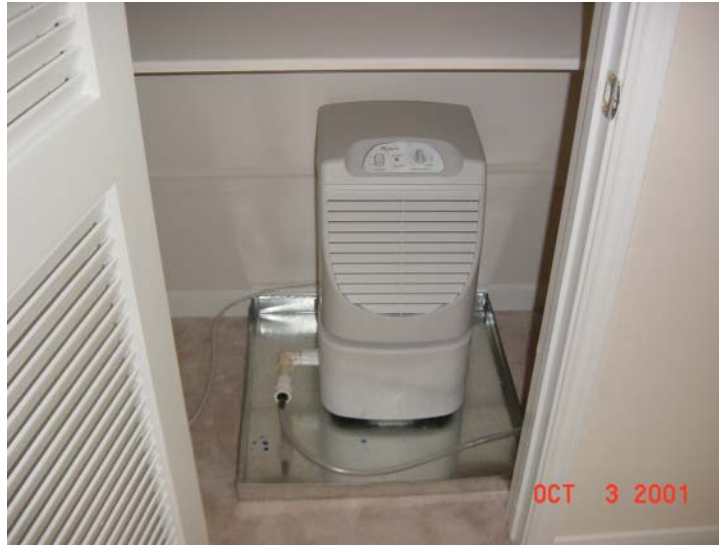
Figure A-1a. Photograph of stand-alone dehumidifier in hall closet with louvered door system
