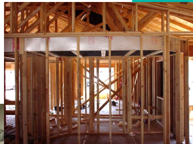
Dropped soffit in hallway
