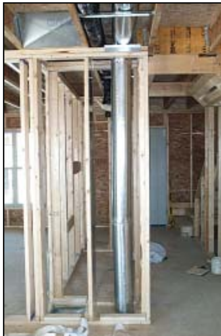
Figure I-33. Kitchen supply duct in central chase
