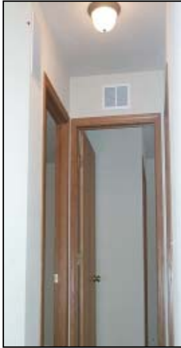
Figure I-35. Second-floor high central return and over-door transfer grille
