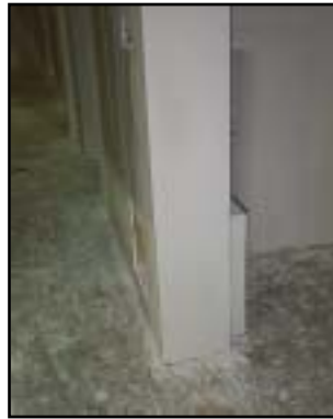
Figure I-50. Central Return in Hall
