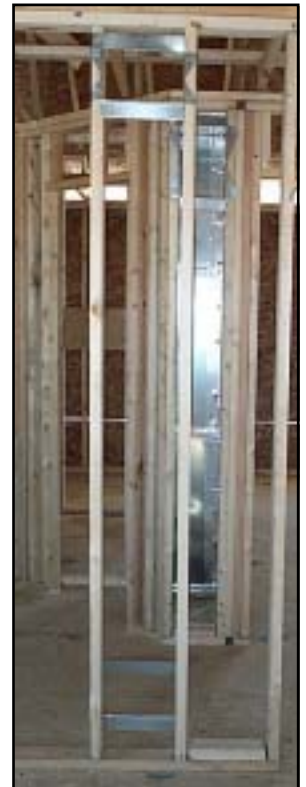
Figure I-34. High/low transfer grille
