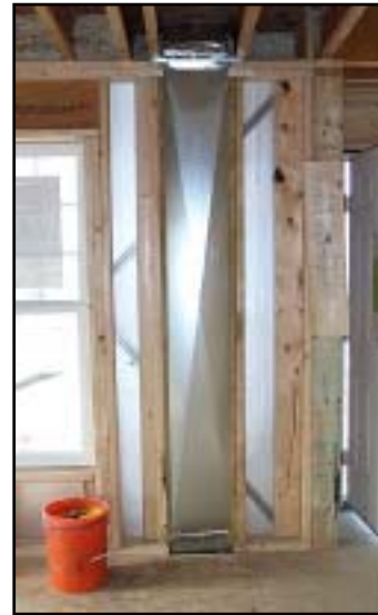
Figure I-25. Supply ducts in exterior walls
