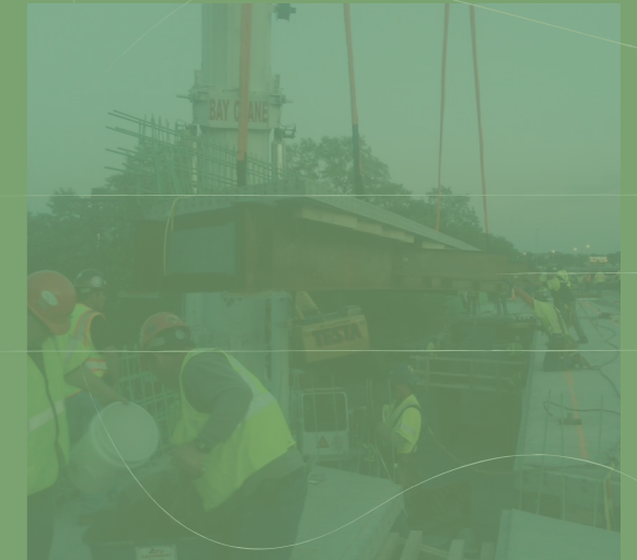
MassDOT Fast 14 Project replaced fourteen bridge superstructures in one construction season using PBES.
