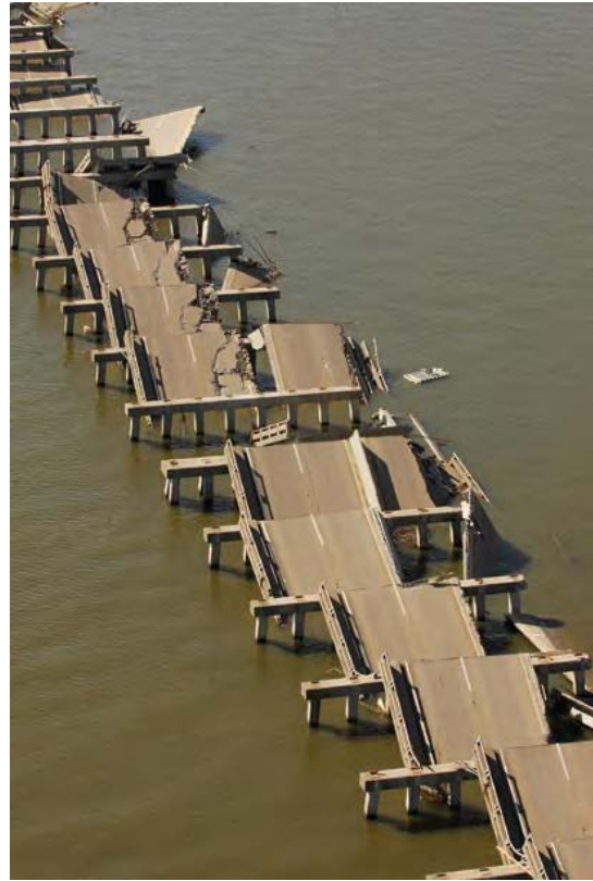
Hurricane Damage from Wave Action to Highway 90 in Bay St Louis, MS (Illinoisphoto.com)
