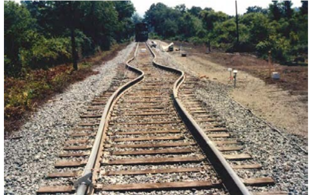
Rail Buckle from High Heat (Photo source DOT Volpe)
