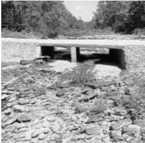
Deceptive innocence. What may look benign—like this box culvert—can keep small fish from reaching all the necessary habitats. FWS photo.
