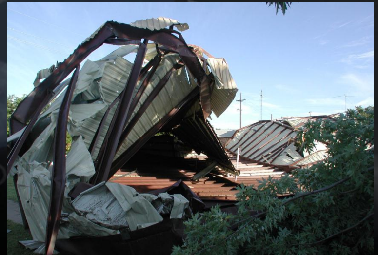
Tornado damage near Ralls, TX – May 12, 2005
