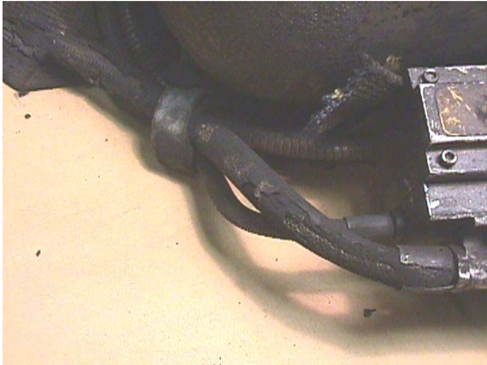
Figure 19 – Unit #1 Low Pressure Hose
