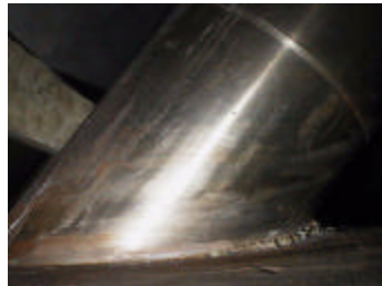
Figure 14 - CRDMP No. 75 L-15 Conoseal CRDM Column at Penetration to RPV Head Interface Side View ( After Cleaning )
