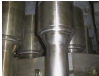
Figure 12 - CRDMP No. 75 L-15 Conoseal/CRDM Column (After Cleaning)
