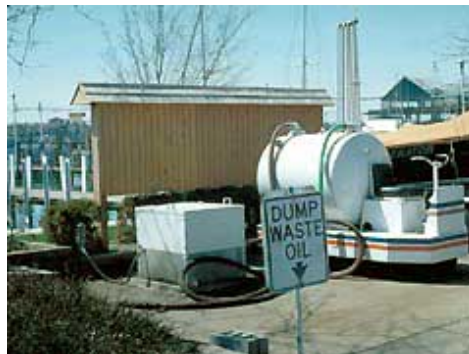
Pump-out stations at marinas such as this one allow boaters to empty their sanitary systems without contaminating the water. Click on image for larger view.
