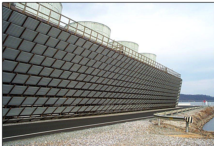
Cooling tower at PBAPS.
