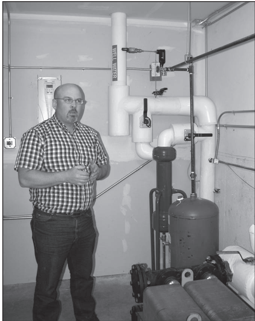
Chuck Bridgeman, Missoula assistant field manager, explains how the ground source heat pump system works. The unit in the foreground is the actual “heat exchanger.”
