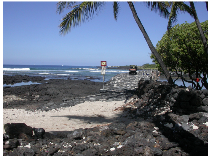
Park staff repair the storm-damaged Kaloko fishpond wall at Kaloko-Honokohau National Historic Park, Hawaii
