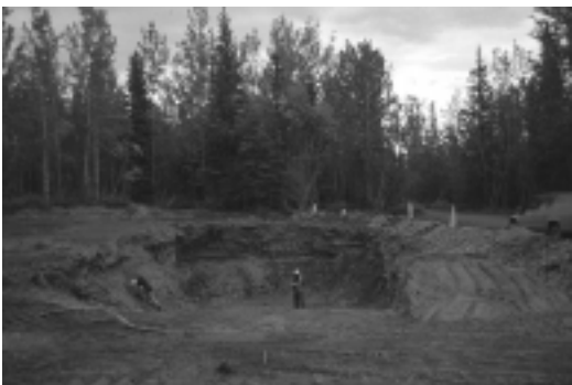
Alaska Department of Transportation gravel extraction along the McCarthy Road. The McCarthy Road is visible on the right.
