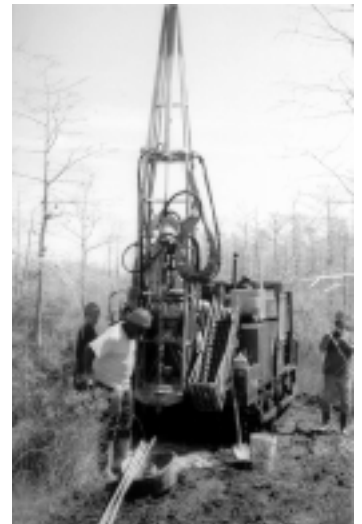
Shothole drilling for 3D seismic survey in Big Cypress National Preserve, Florida.
