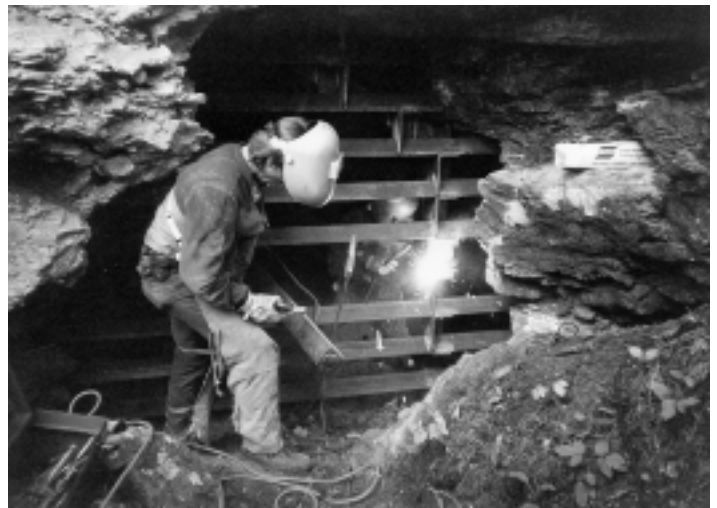
Installation of a gate closure specifically designed to allow bat access while reducing safety concerns at Buffalo NR.
