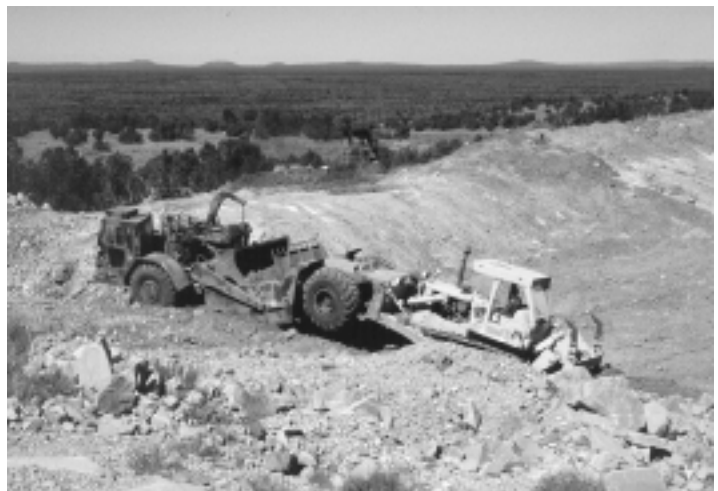
The use of heavy equipment enabled the establishment of a stable surface that conforms to the surrounding landscape at El Malpais NM.
