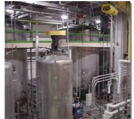
Large-scale anaerobic fermentation and liquefaction equipment in starch pilot plant
