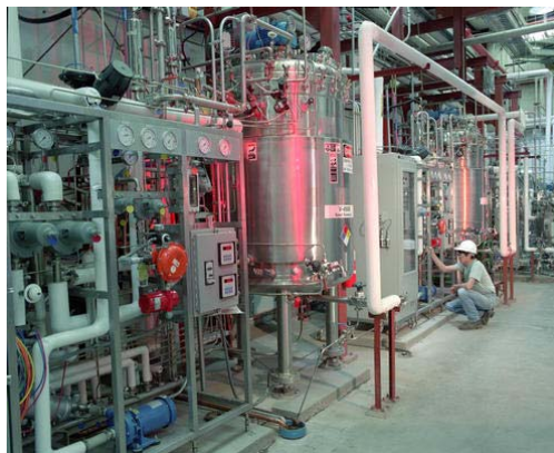
Integrated pilot plant for lignocellulosic biomass processing.
