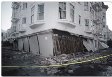
Buildings in the Marina District of San Francisco were badly damaged in the 1989 Loma Prieta earthquake. “Soft story” buildings, typically with parking on ground floor, like the one pictured here, are common throughout the Bay Area and are particularly at risk when exposed to strong shaking. (USGS photo)
