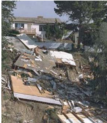
Landslides —Earthquakes can trigger landslides that damage roads, buildings, pipelines, and other infrastructure. Steeply sloping areas underlain by loose or soft rock are most susceptible to earthquake-induced landslides. This home was destroyed when the hillside beneath it gave way following the 1994 magnitude 6.7 Northridge earthquake (FEMA photo).
