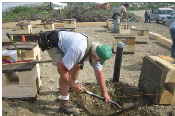
Eagle, AK, July 29, 2009 - Volunteer helps to prepare the foundation to a new home in Eagle, AK, for a disaster survivor. (Photo: Ben Brennan/FEMA)
