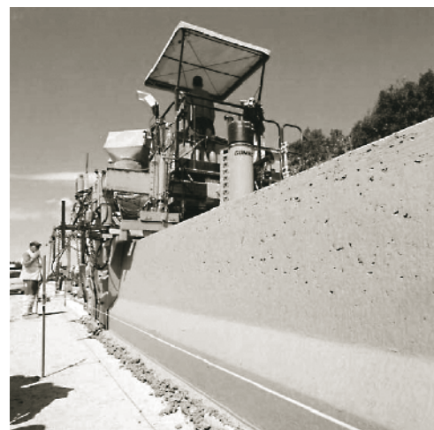
Figure 46. Slipform paving of the safety barriers on the E40/A10 CRC overlay project.
