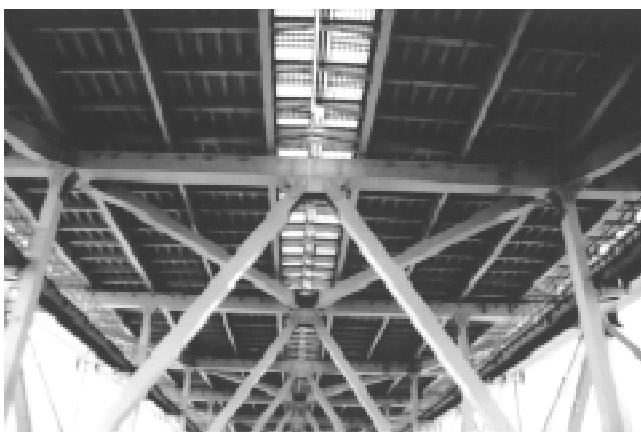
Figure 4. Vents to equalize air pressure on the Akashi-Kaikyo Bridge.
