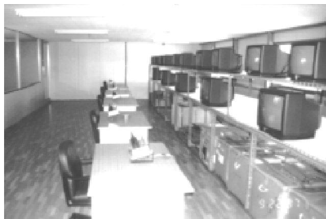
Figure 24. Control room for excavation in pneumatic caissons.
