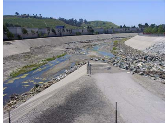
Flood Control—San Juan/Arroyo Trabuco Creeks
