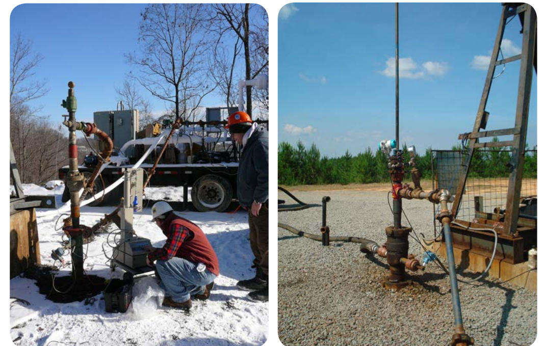
Injection operations at the Central Appalachian (left) and the Black Warrior Basin (right) project sites.
