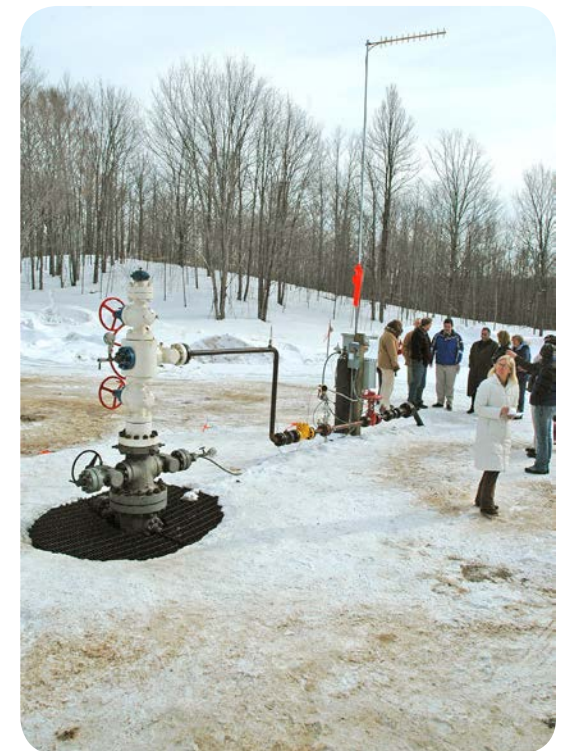
Visitors examine an MRCSP CO 2 injection well in action.
