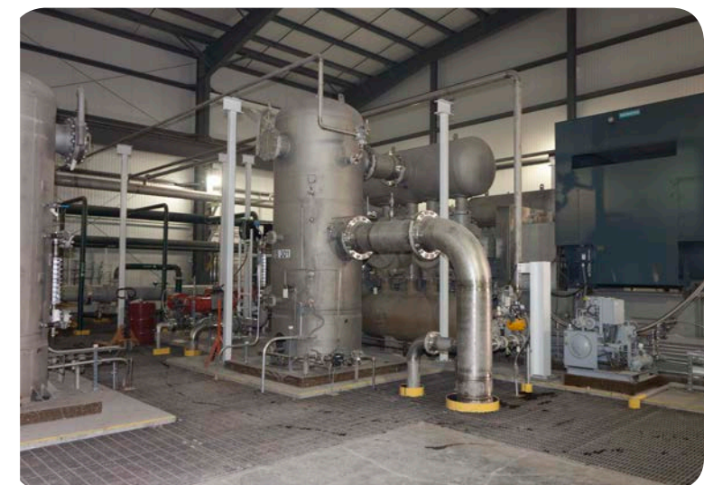
Inside of the IBDP CO 2 compression-dehydration facility.
