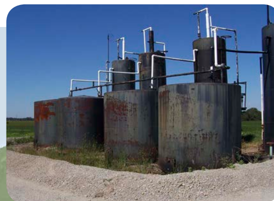
Oil tank battery.
