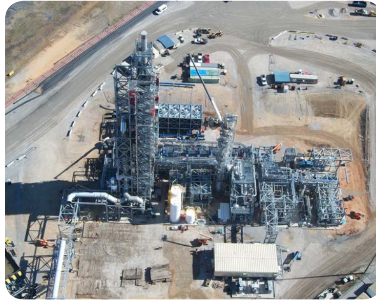
CO 2 capture facility at Plant Barry. (Photo courtesy of Southern Company)
