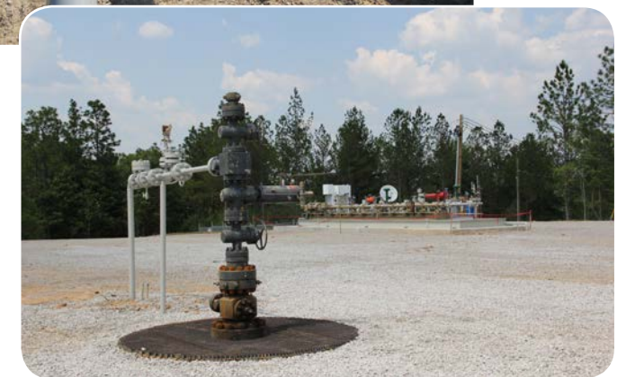
CO 2 injection well at Denbury's Citronelle oil field. (Photo courtesy of SSEB)
