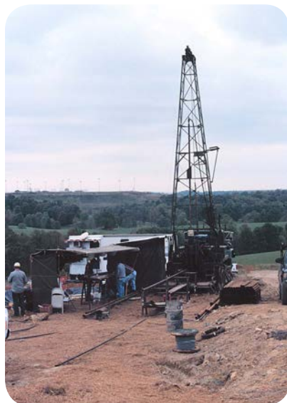
Coalbed methane wells like the one shown here are present in much of the MRCSP region.
