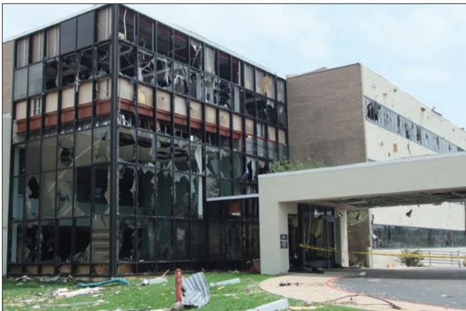
The main entrance and lobby of the St. John's administrative building shows the remnants of shattered glass and flying debris.
