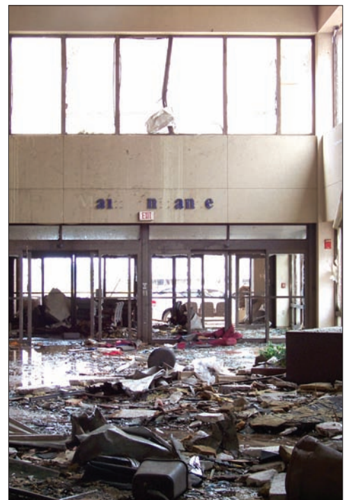
The interior of St. John's main entrance provides an example of the destruction inside the hospital.
