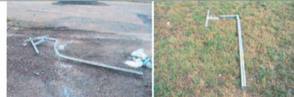
Figure 1. Crash performances for H-base sign structures.
