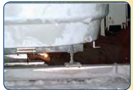
On November 28, 2007, ACRF operations and engineering staff braved -15 degrees F weather to install the new radar antenna at Barrow. Here, ACRF lead engineer Kevin Widener goes gloveless to securely fasten all the tiny connecting screws and bolts—brrrrr!
