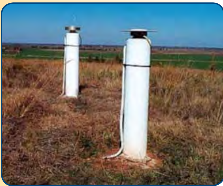
GPS receivers are installed at all the extended facilities throughout the SGP domain.
