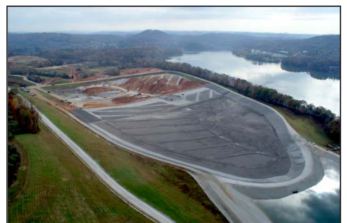
This aerial view shows the progress made on the lined gypsum pond at the Kingston Fossil Plant.
