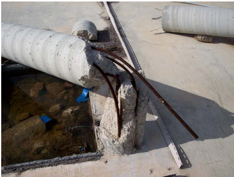
Figures 38 and 39. Reinforced Concrete Columns Failure
