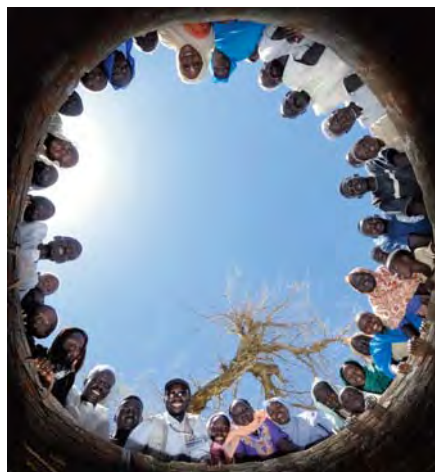
Residents of a displaced persons camp in West Darfur, Sudan, look down a well they helped build.
