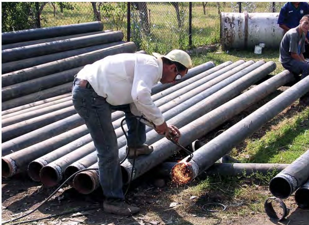
A village in Armenia awaits its first running water as a worker makes final preparations to pipes that will deliver water from a nearby source.
