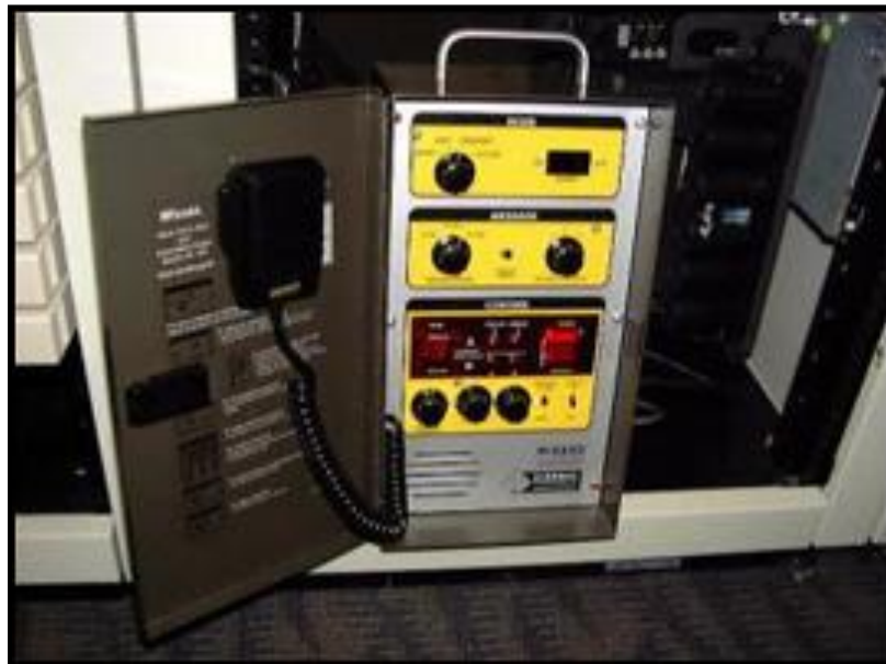
FIGURE 2.10 The installation of CB Wizard alert system (Trimarc)
