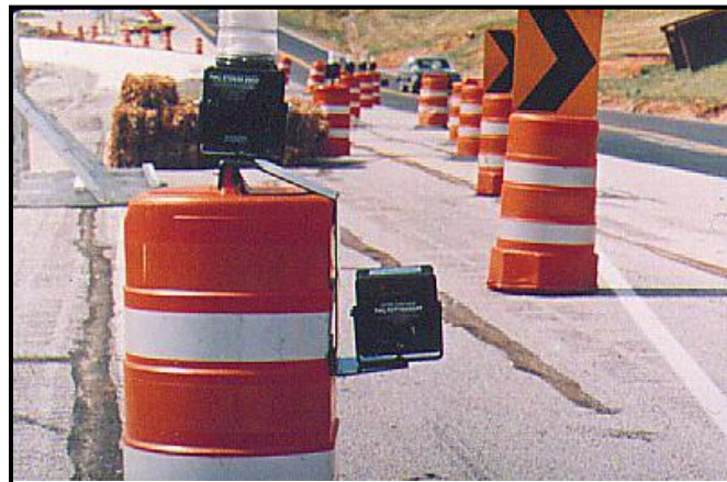
FIGURE 2.3 The installation of microwave intrusion alarm (Hatzi 1997)
